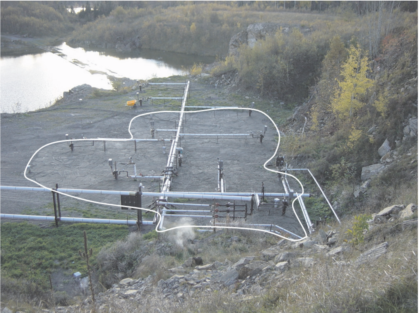
Figure 5.4-1. Location of the concrete seal placed over the eastern part of the site in mid-October.
