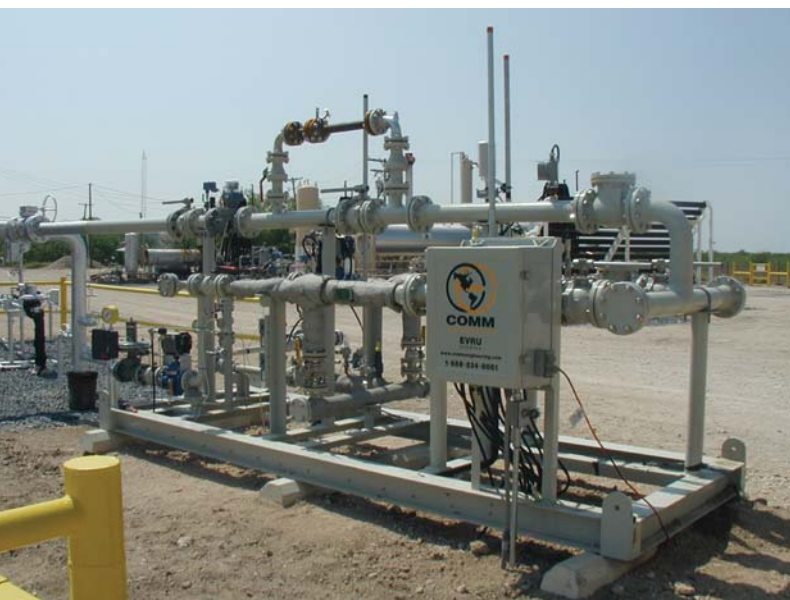
The COME Engineering EVRU installed
