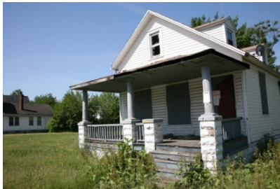
In Cleveland, Ohio (shown above) a dilapidated house next to a vacant lot (left); a vacant lot post-demolition (center), and a vacant lot after extensive post-demolition debris removal, soil management, and plantings (right).
