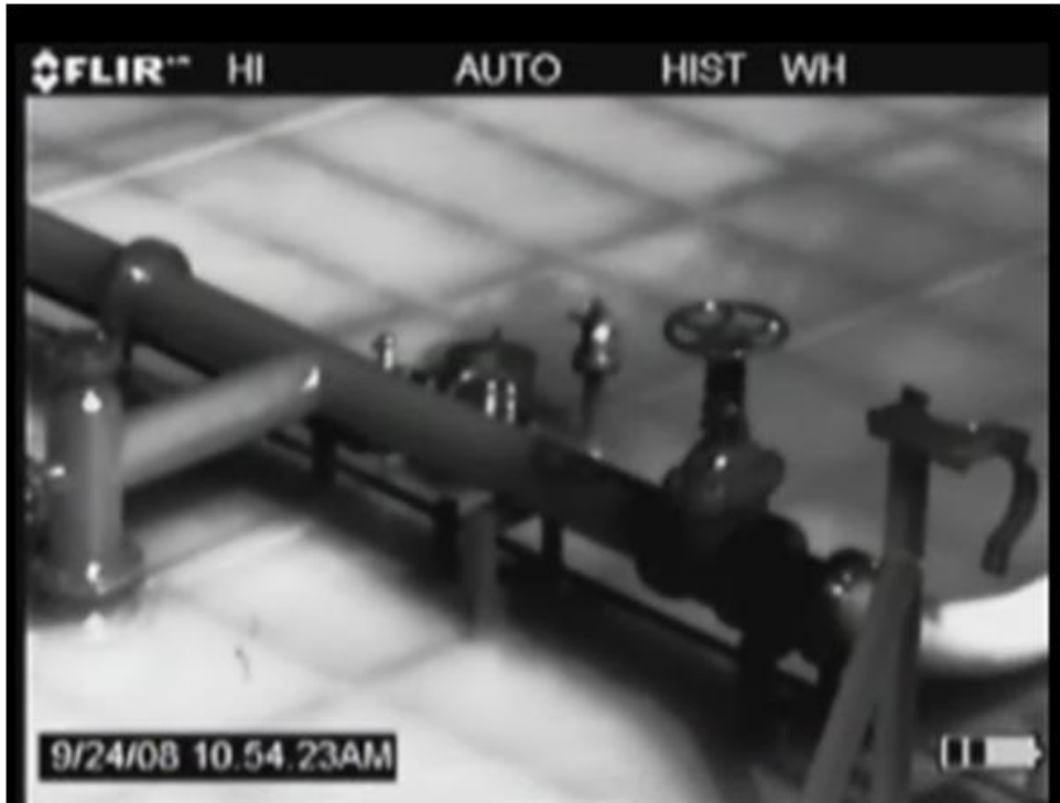
Figure D-1. Leak from Barge L1 (captured while barge in lock)
