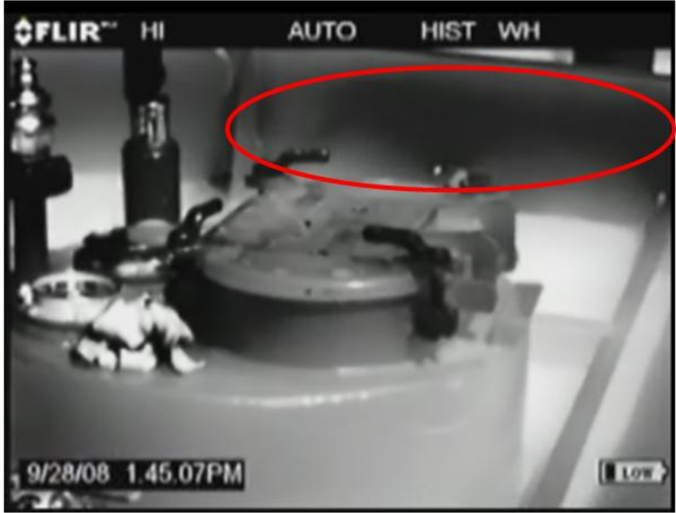
Figure D-28. Leak from Barge G8 (captured while onboard barge)
