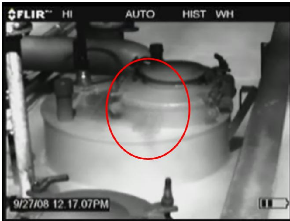
Figure D-22. Leak from Barge G6 (captured while onboard barge)
