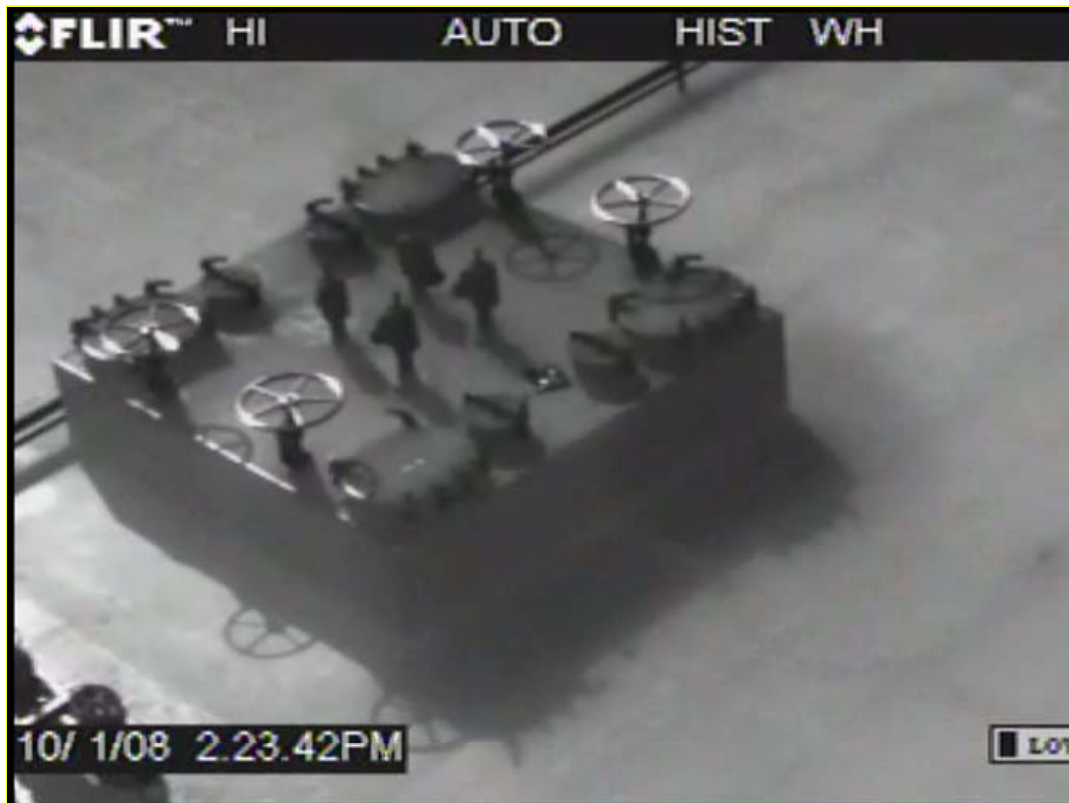
Figure G-5. Screenshot from FLIR Camera Showing Leak from 10/1/ 2008, Event #6
