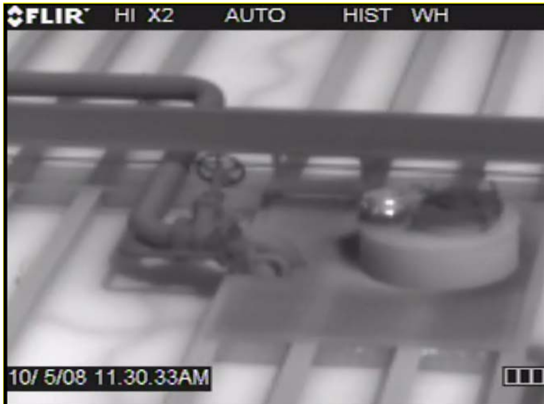
Figure G-9. Screenshot from FLIR Camera Showing Leak from 10/5/ 2008, Event #2
