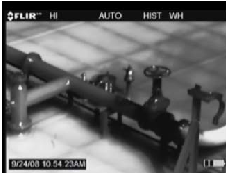
Figure 4-1. Screenshot from FLIR Camera Showing Leak from 9/24/ 2008, Event #1
