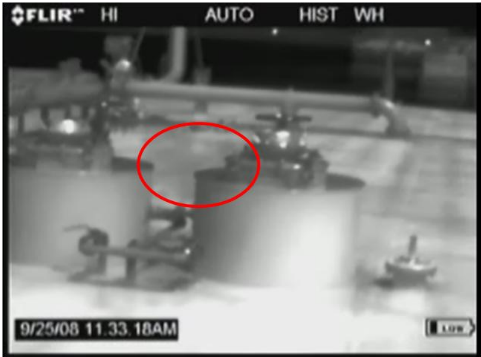
Figure D-9. Leak from Barge G2 (captured while onboard barge)
