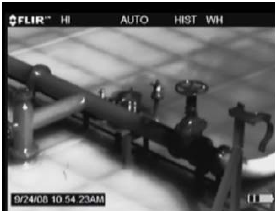
Figure G-2. Screenshot from FLIR Camera Showing Leak from 9/24/ 2008, Event #1
