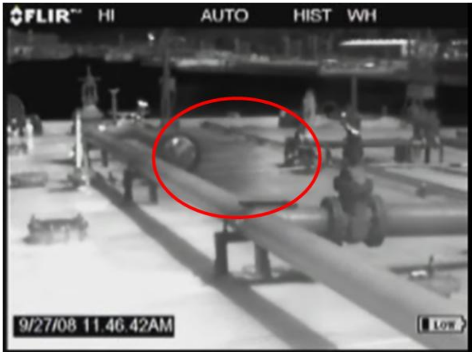
Figure D-19. Leak from Barge G6 (captured while onboard barge)
