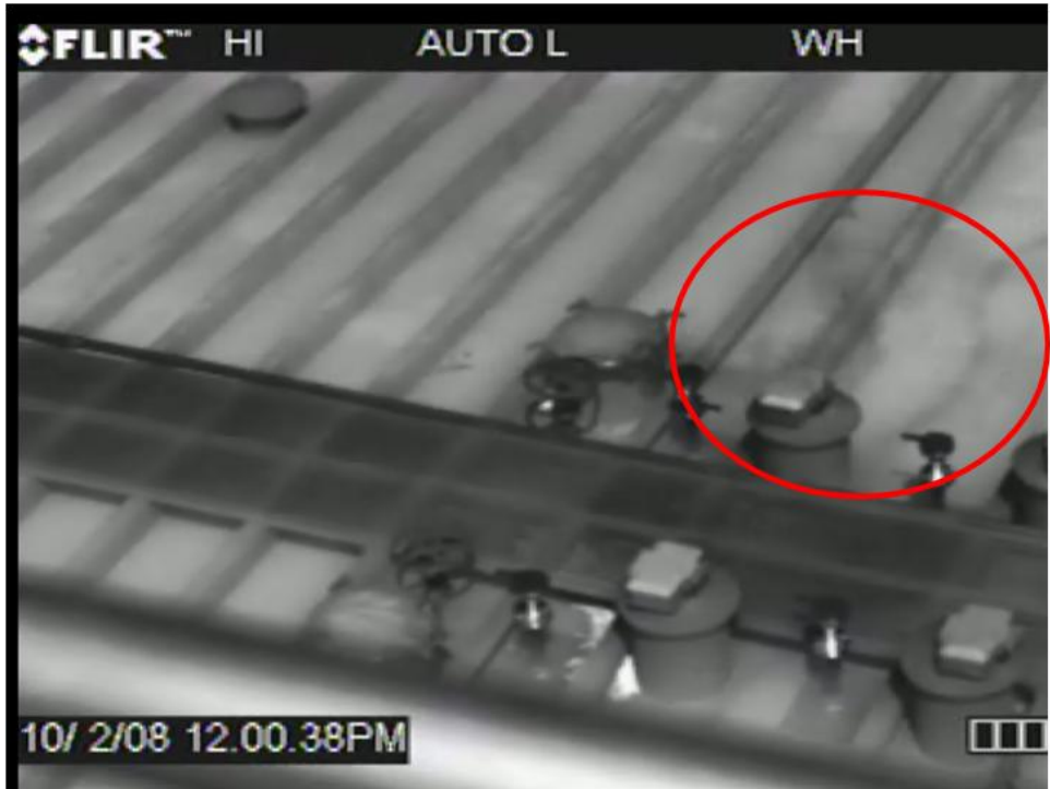
Figure E-12. Leak from Hatches 10/2
