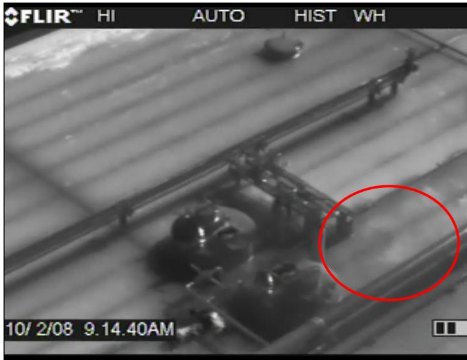
Figure E-7. Leak from Hatch 10/2
