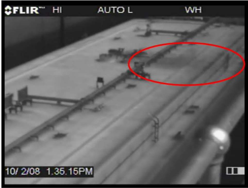
Figure E-13. Leak from Hatches 10/2
