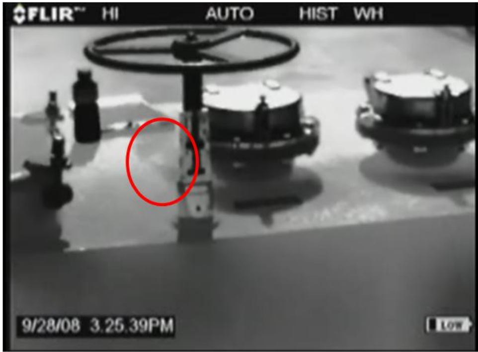
Figure D-38. Leak from Barge G8 (captured while onboard barge)
