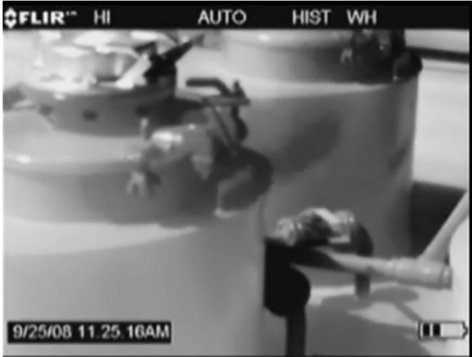
Figure D-7. Leak from Barge G2 (captured while onboard barge)
