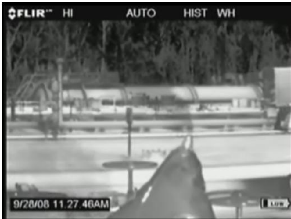
Figure D-26. Leak from Barge G7 (captured while onboard barge)
