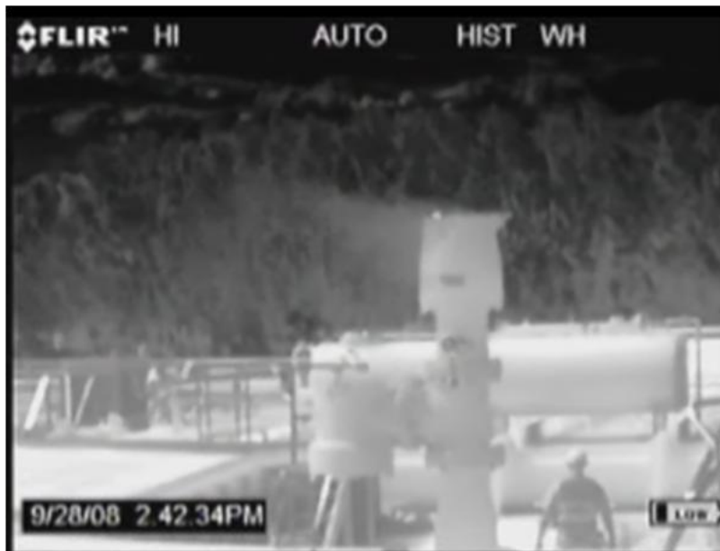
Figure 3-14. Leak from Pressure Relief Valve on Barge G8- Mass Leak 5.78 g/s
