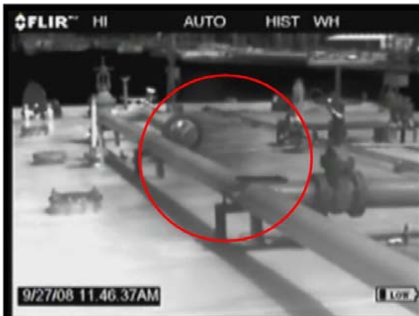
Figure 3-11. Leak from Vent on Barge G6- Mass Leak 1.45 g/s
