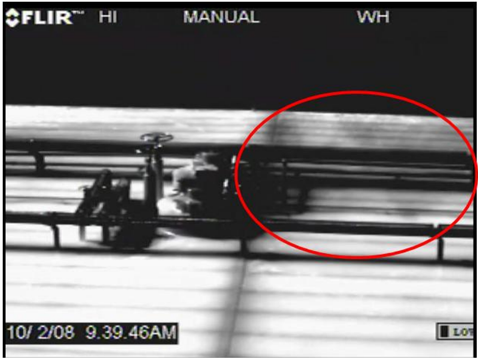
Figure E-11. Leak from Valve 10/2
