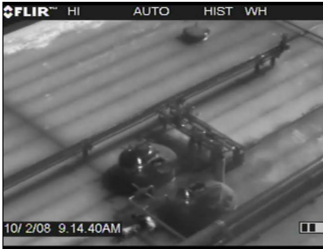
Figure 4-4. Screenshot from FLIR Camera Showing Leak from 10/2/ 2008, Event #3
