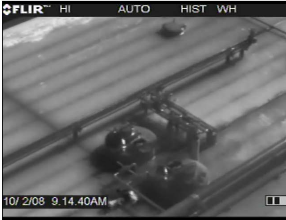
Figure G-6. Screenshot from FLIR Camera Showing Leak from 10/2/ 2008, Event #3
