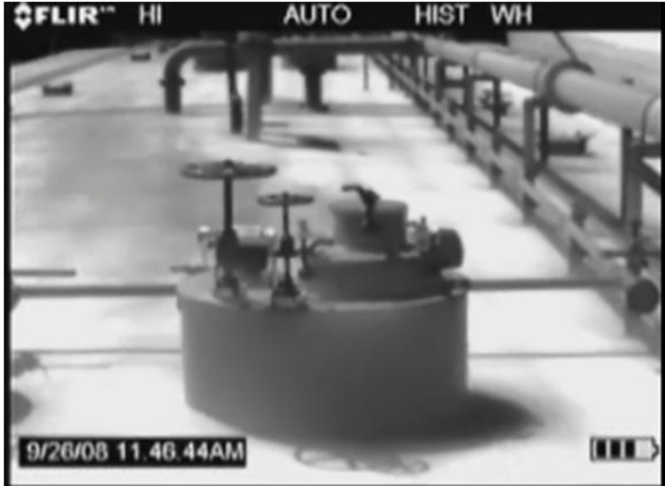
Figure D-18. Leak from Barge G5 (captured while onboard barge)
