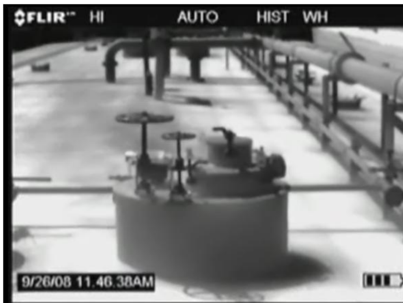
Figure 3-9. Leak from Ullage Hatch on Barge G5- Mass Leak 0.73 g/s
