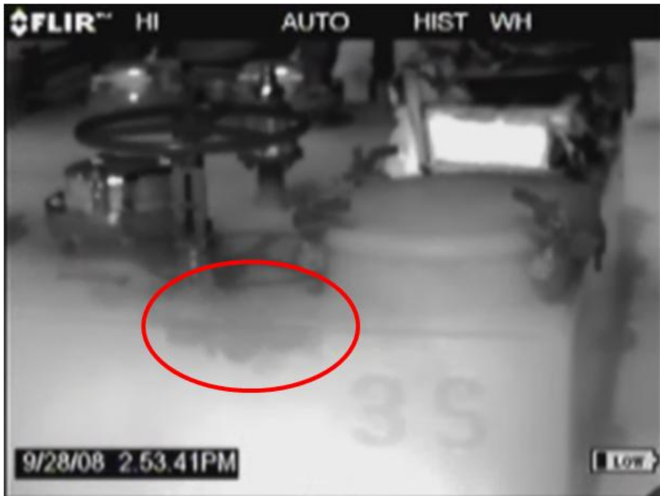
Figure D-33. Leak from Barge G8 (captured while onboard barge)
