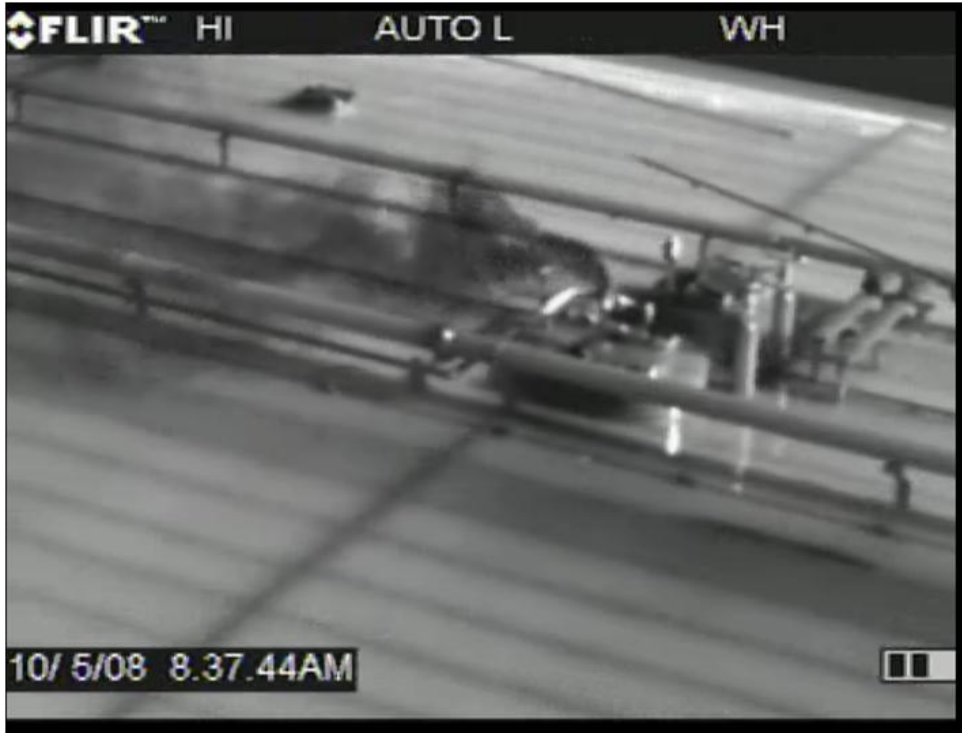
Figure E-14. Leak from Valves 10/5
