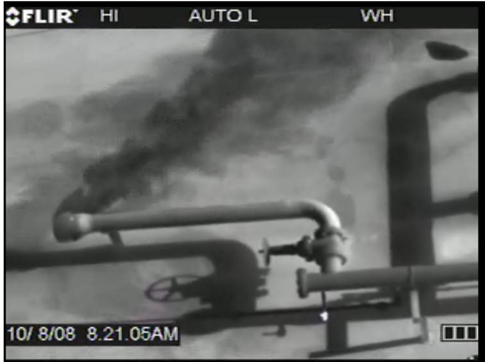
Figure E-16. Leak from Pipes 10/8
