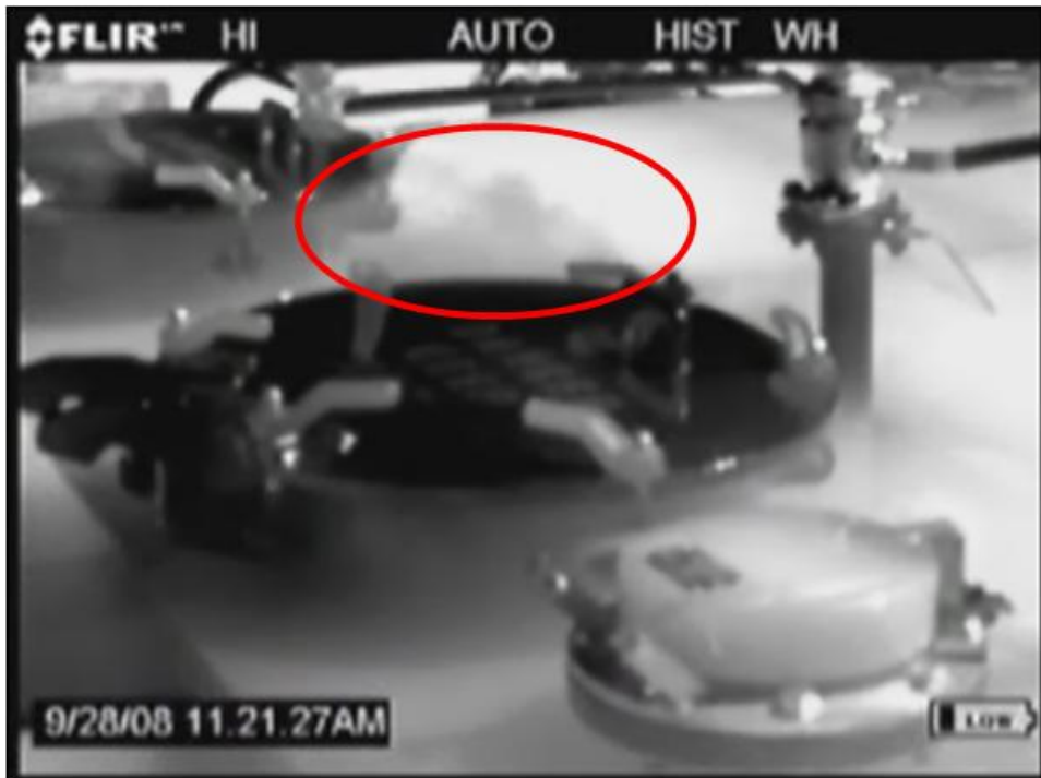
Figure D-25. Leak from Barge G7 (captured while onboard barge)
