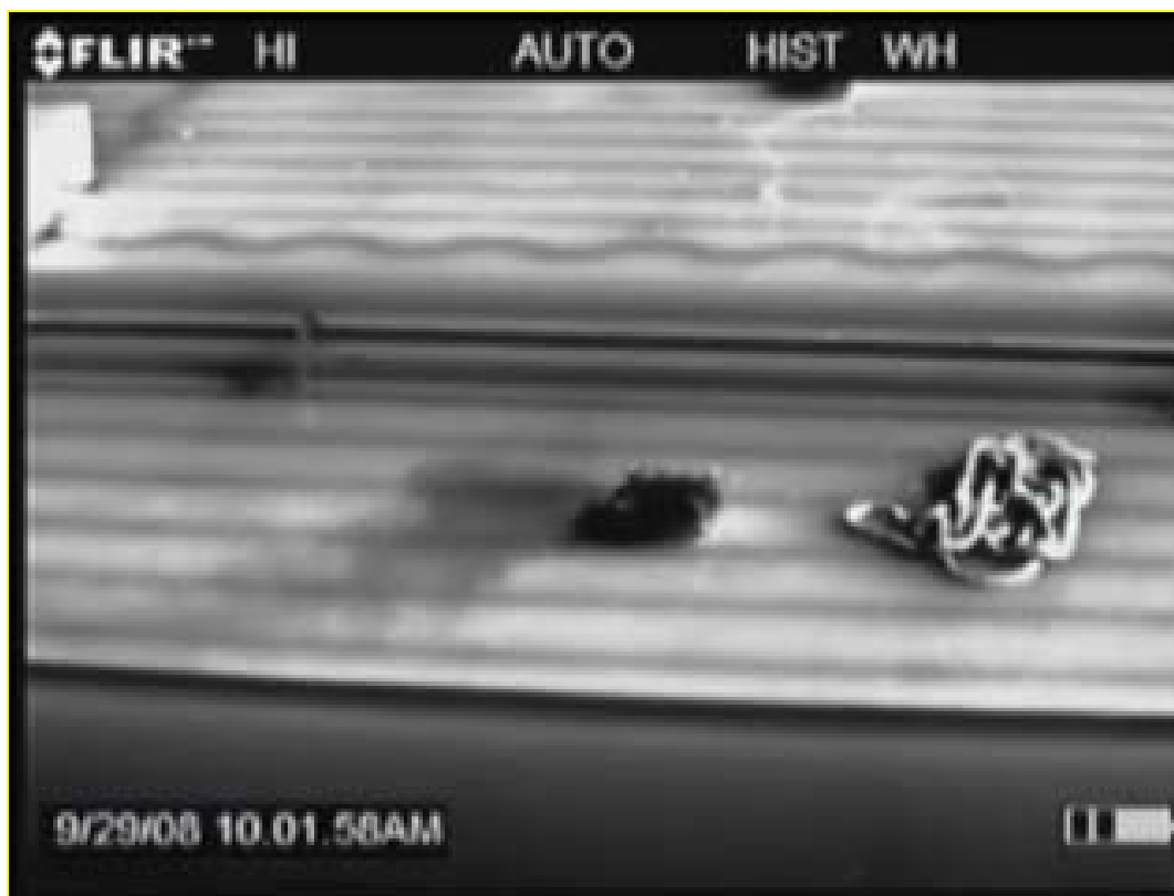
Figure G-3. Screenshot from FLIR Camera Showing Leak from 9/29/ 2008, Event #2
