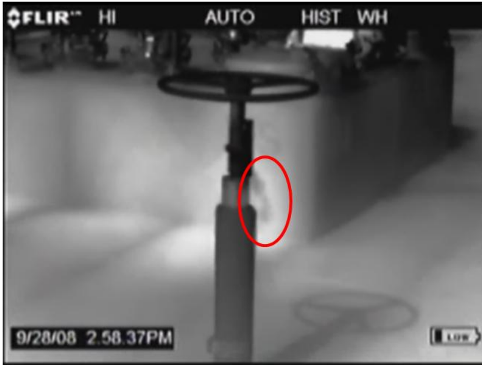
Figure D-35. Leak from Barge G8 (captured while onboard barge)
