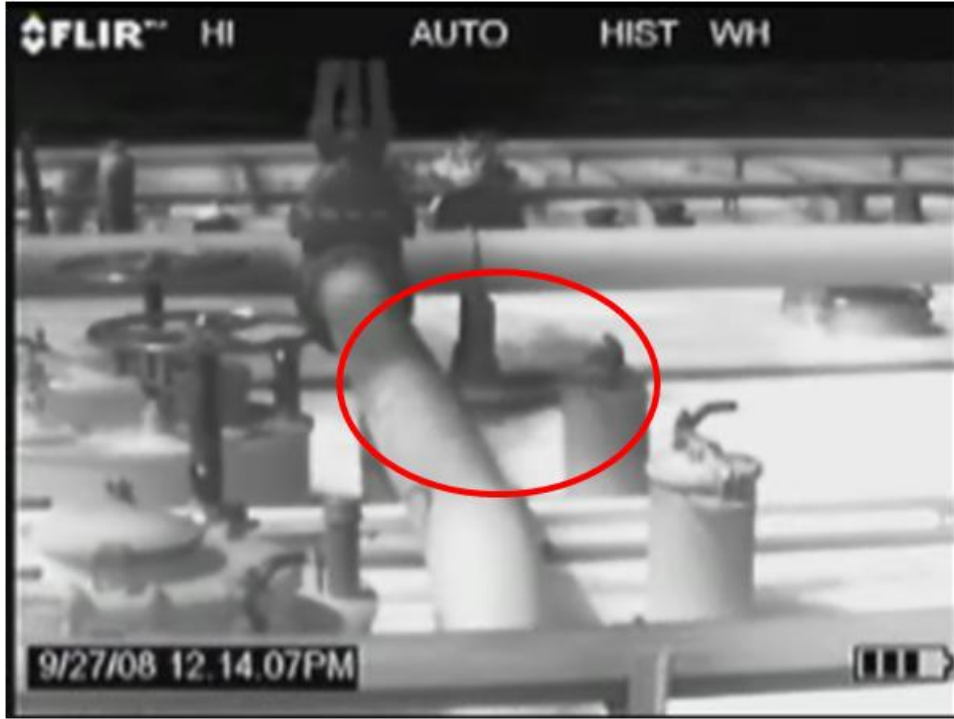
Figure D-21. Leak from Barge G6 (captured while onboard barge)
