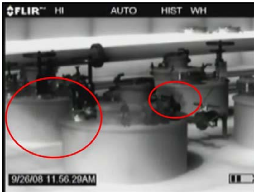
Figure 3-10. Leak from Ullage Hatch on Barge G5- Mass Leak 1.43 g/s
