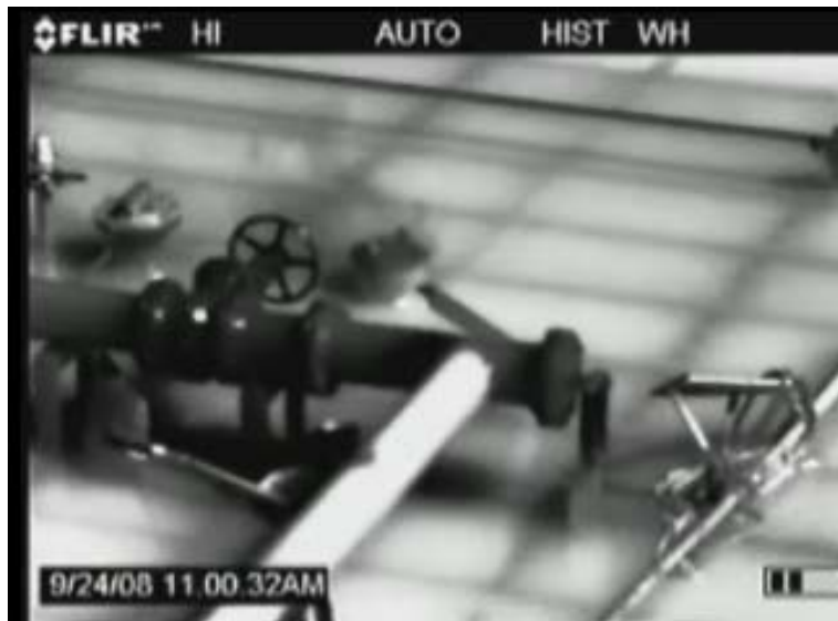
Figure 3-16. Example #2 from LSI Ground Survey – Leaking Valve on Barge L2- Total Mass Emission from Barge 0.521 g/s
