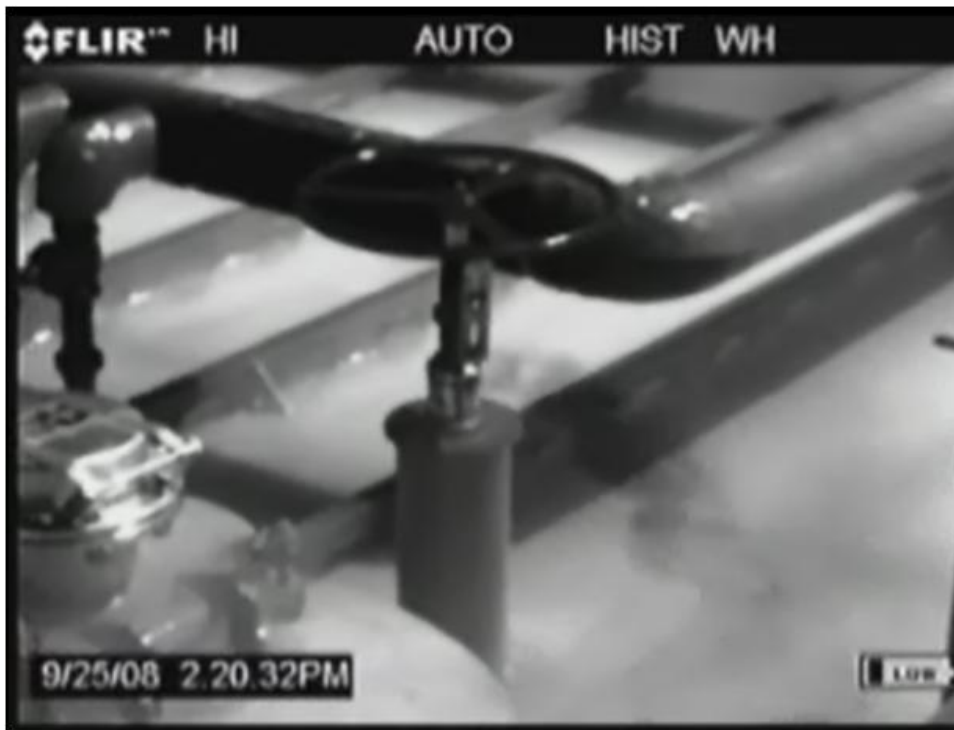
Figure D-16. Leak from Barge G3 (captured while onboard barge)
