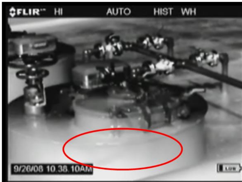
Figure 3-6. Leak from Ullage Hatch on Barge G4- Mass Leak 0.31 g/s
