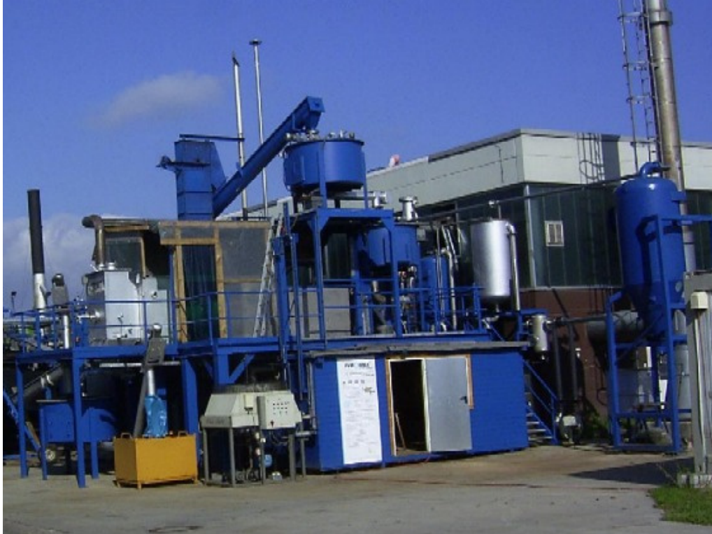
Figure 9 - Pryomex Ultra High Temperature gasifier in Munich, Germany 20
