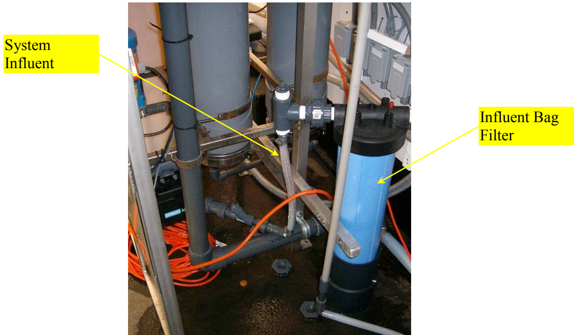
Figure 2-3. ITT Fyne Technology System Influent 3-Foot Module
