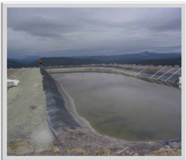
Fig. 14. Constructed biochemical reactor (BCR)
