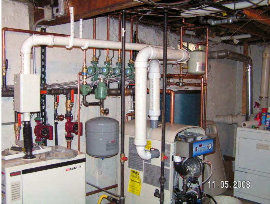
Figure 1-1. Freewatt Hydronic System Tested in Lake Rononkoma, NY
