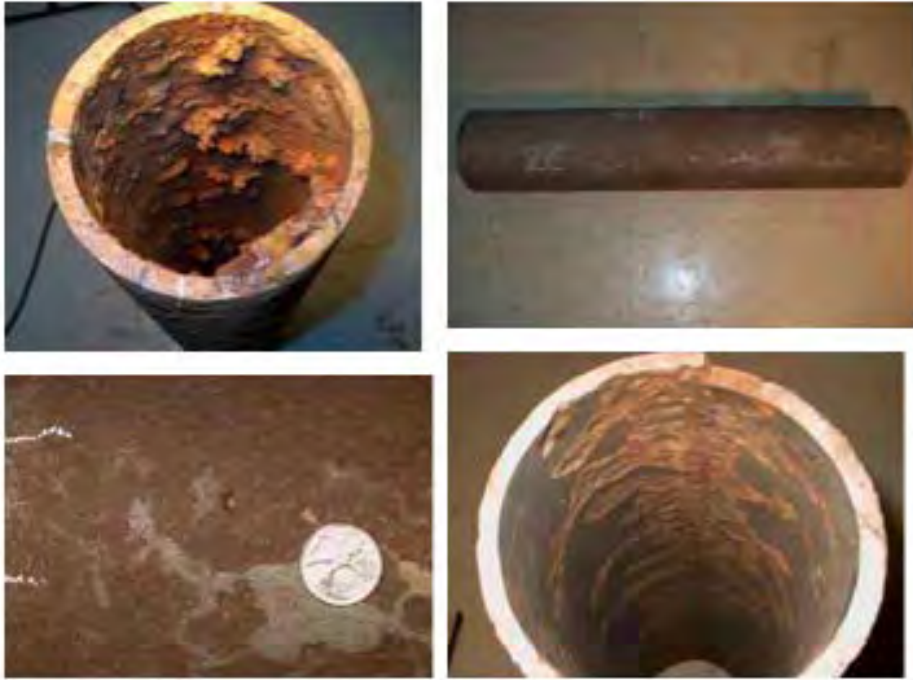
Figure 1: Photos of pipe with 4.2% measured loss
