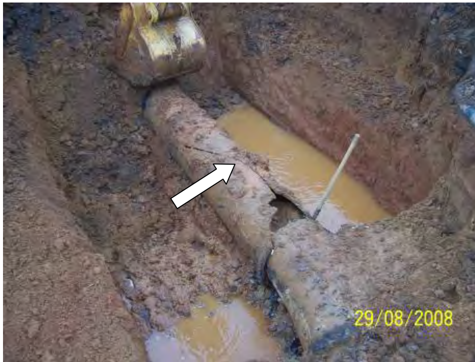
Note arrow pointing to longitudinal propagation of crack
