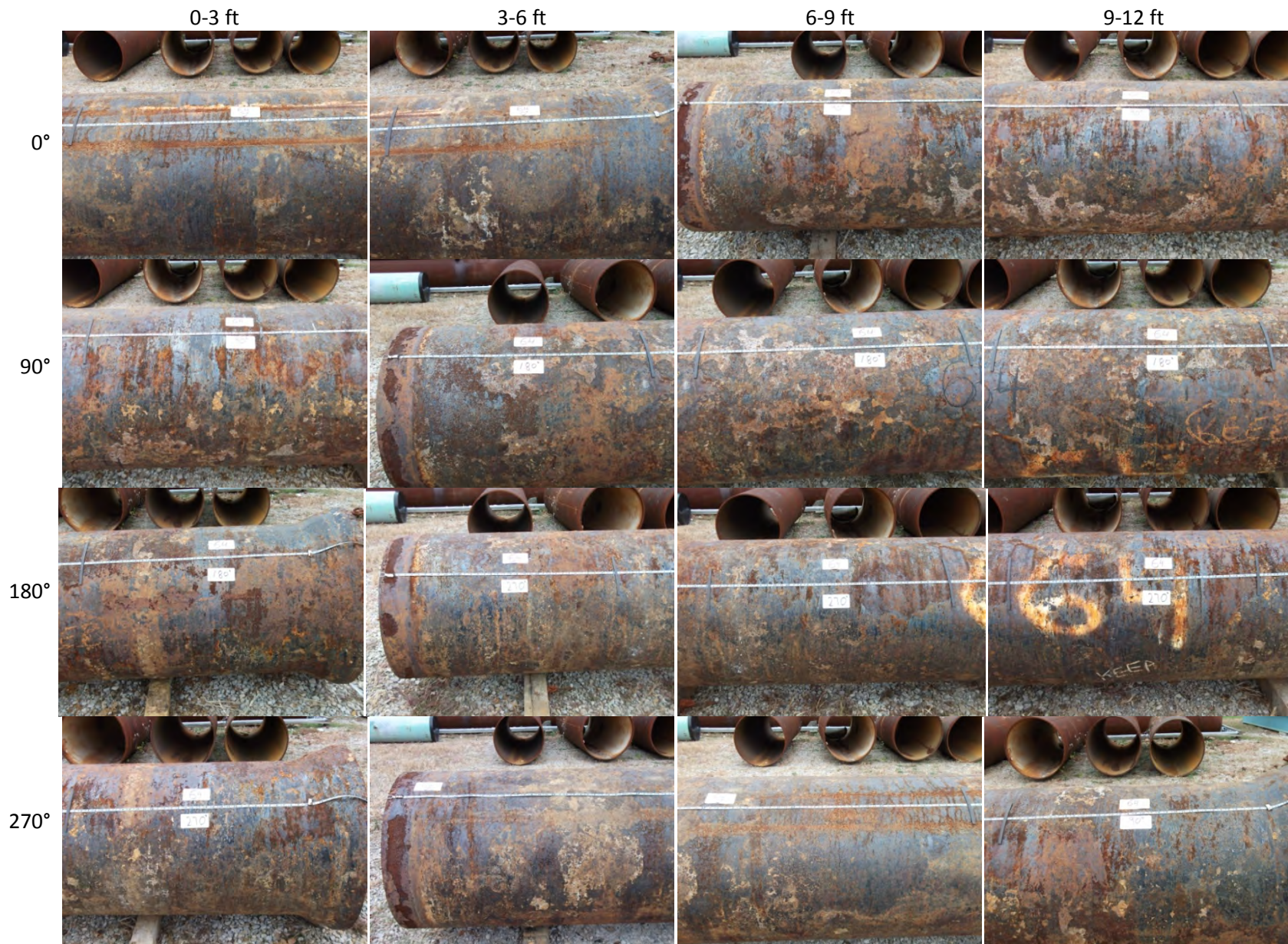
Figure A-64(1). Pipe 64 as Removed from Site
