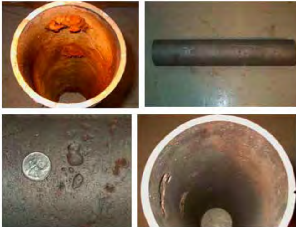
Figure 2: Photos of pipe with 8.9% measured loss
