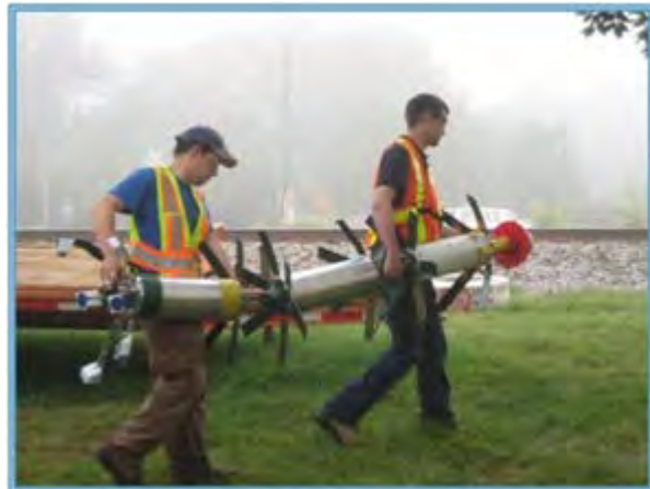
Carrying the PipeDiver tool ready to be installed into the insertion tube.
