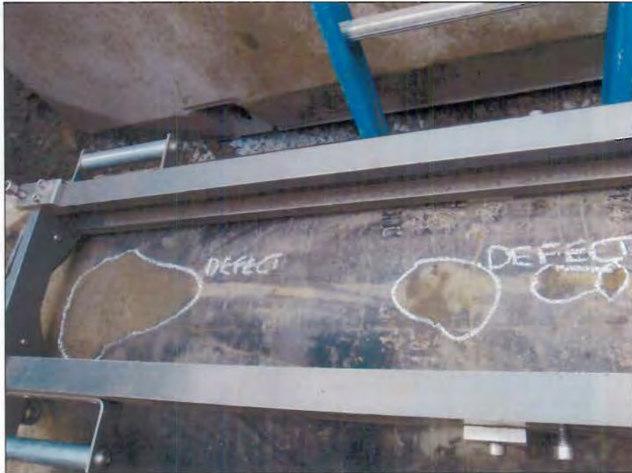
FIGURE A5.15 - PHOTOGRAPH OF DEFECTS IDENTIFIED ON THE PIPE
