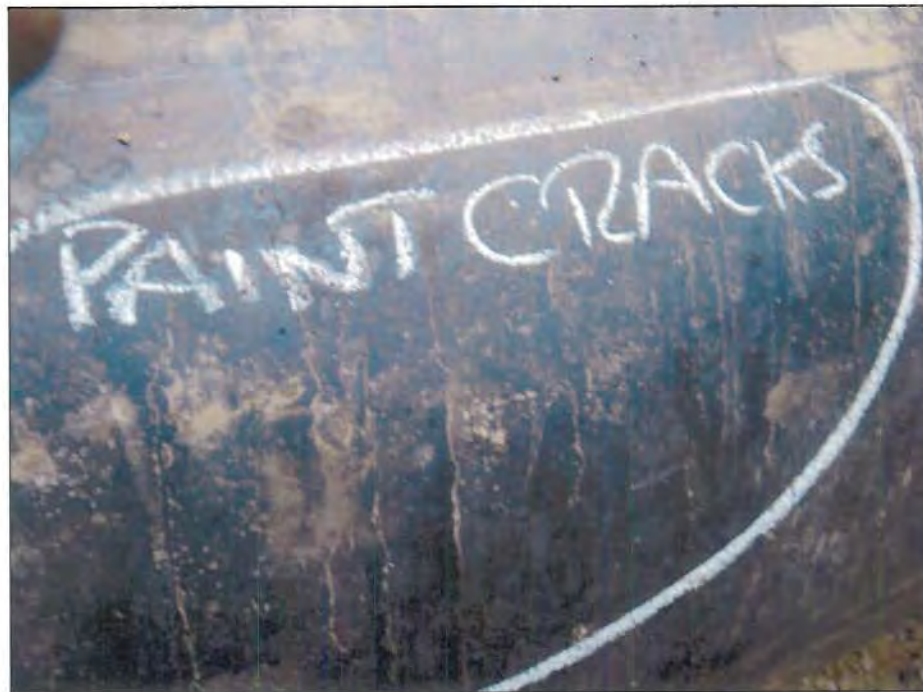
FIGURE A5.16 - PHOTOGRAPH OF COATING DEFECTS
