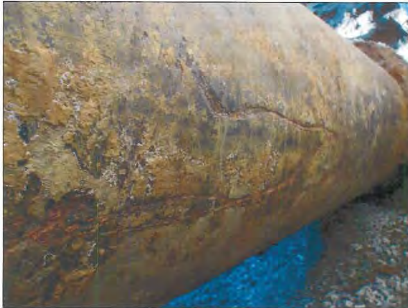
FIGURE 4.5 - AREA OF MECHANICAL DAMAGE
