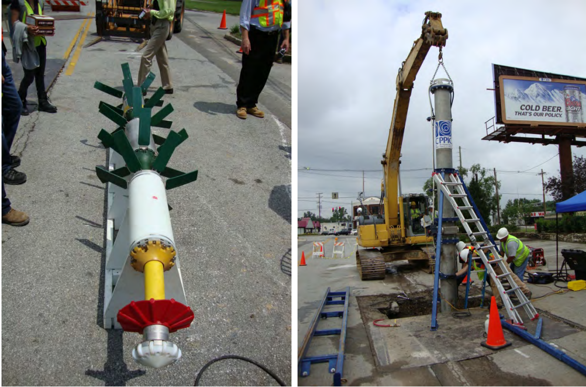
Figure 3-10. PipeDiver® Inspection Vehicle (left) and Insertion Tube (right)
