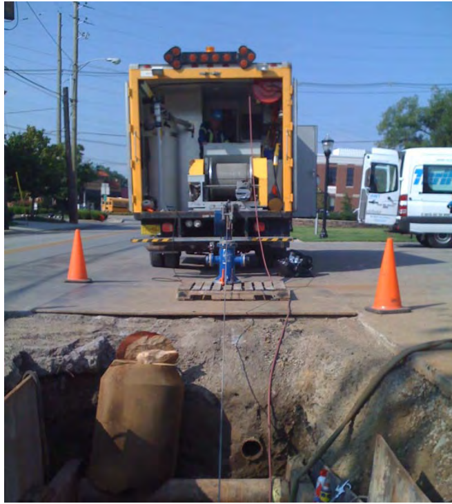
Figure 3-36. Wireline Truck and Hydrant Set-up
