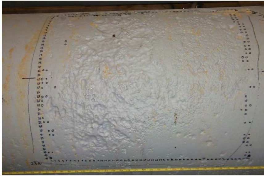
Figure 4-4. Corrosion Area on Pipe 69: 95-in. from the spigot, 129-degrees from the top of the pipe, 27-in. in axial extent and 109-degrees in circumferential extent
