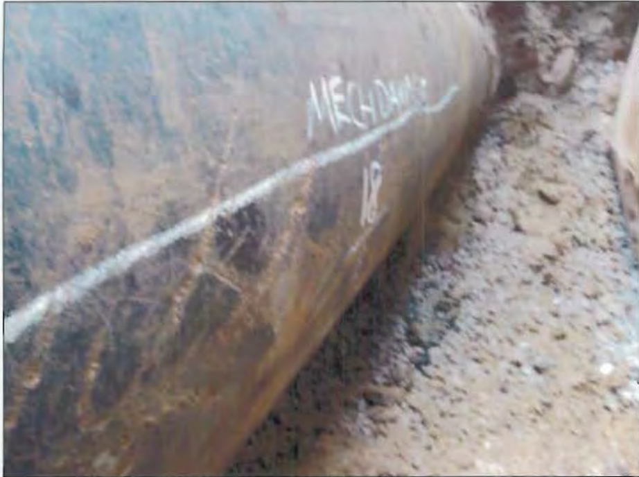
FIGURE A5.17 - PHOTOGRAPH OF MECHANICAL DAMAGE TO THE PIPE
