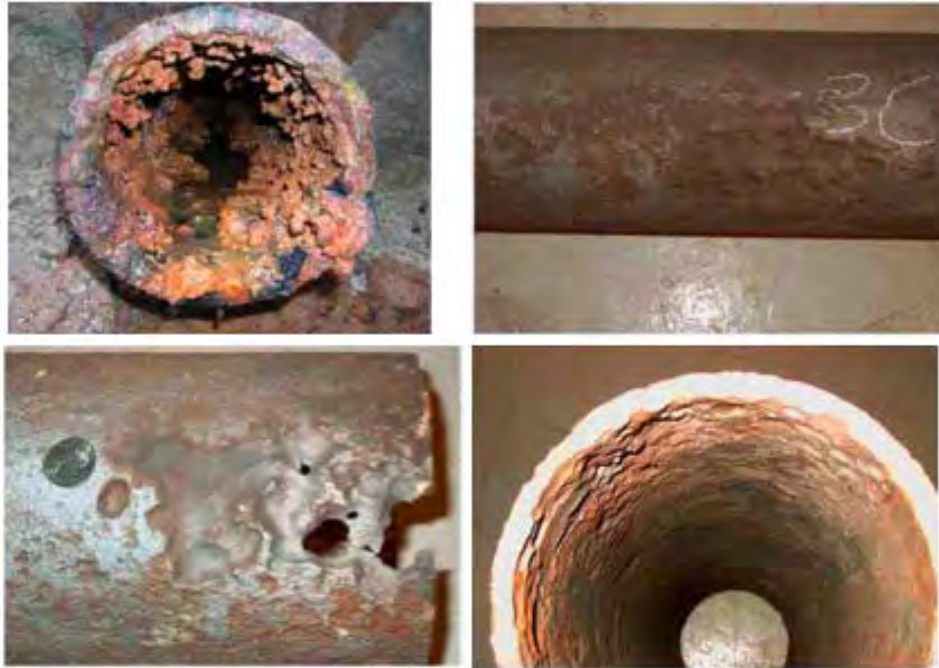
Figure 3: Photos of pipe with 47.3% measured loss
