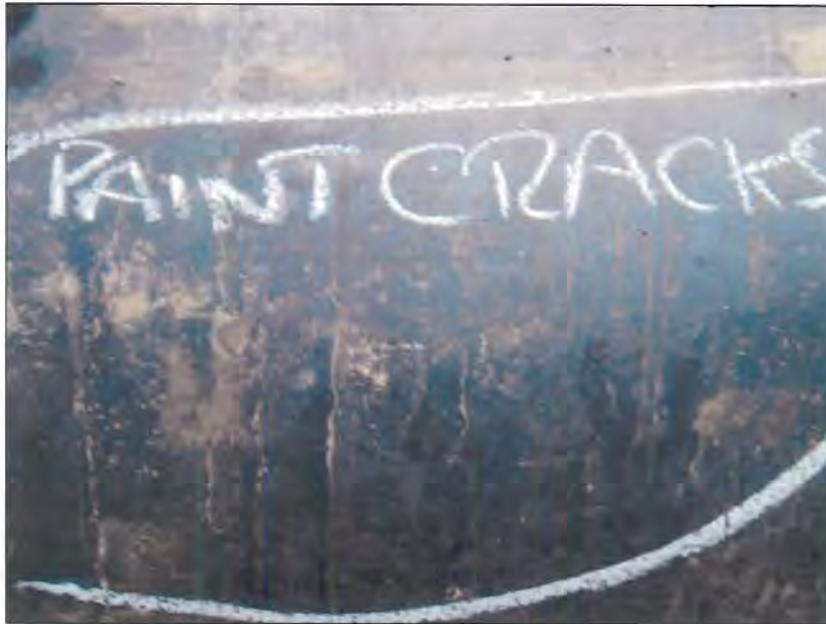
FIGURE 4.11 - PHOTOGRAPH OF COATING DAMAGE
