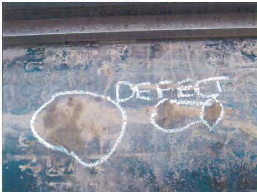
FIGURE 4.12 - PHOTOGRAPH OF EXTERNAL DEFECTS
