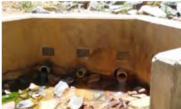
Figure 2. Virginia Canyon (1st and 2nd from left) and Big Five Tunnel (far right) outfalls. Photo by Arcadis.
