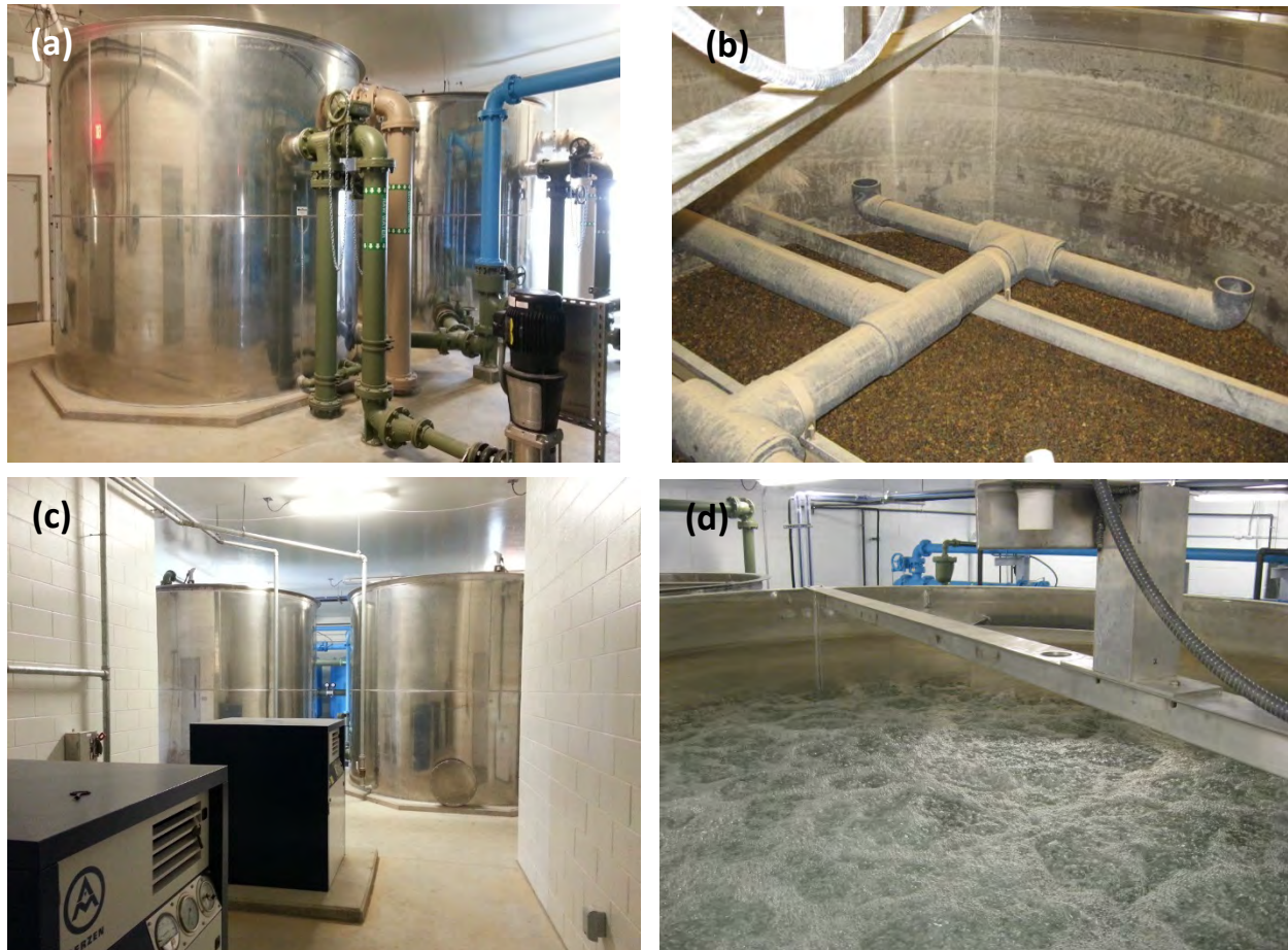
Figure 6. Photographs of (a) aeration contactors, (b) contactor media and piping, (c) aeration contactors and air blowers, and (d) aerated contactor surface.
