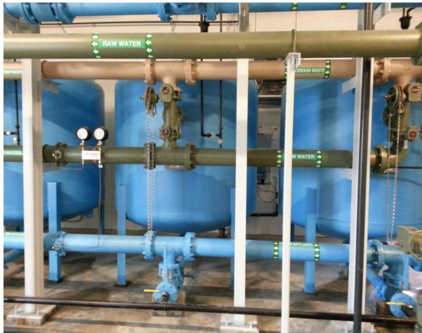
Figure 7. Photograph of pressure filters.
