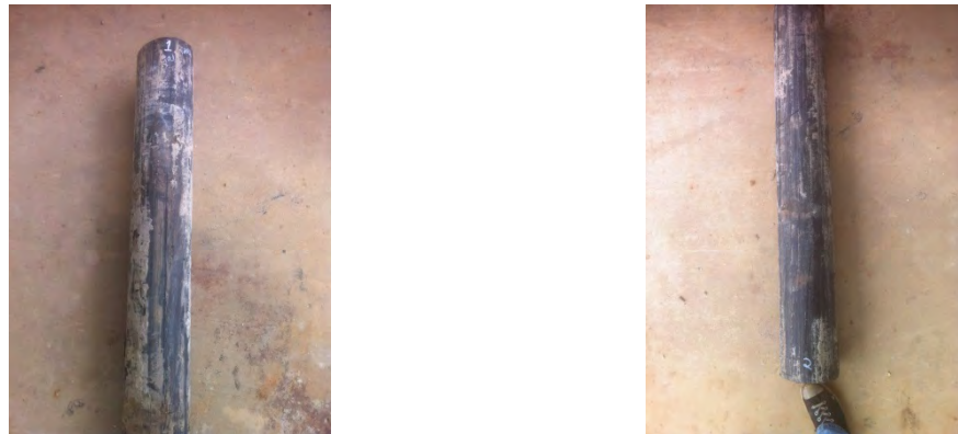
Figure C-50. Houston – Norton Dr.: Images of the Black Polyethylene Slipliner Section Prior to Testing
