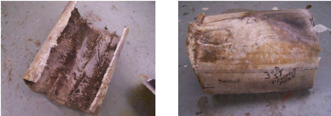
Figure B-66. New York 1: Defective Sample Retrieved from 3rd Street
