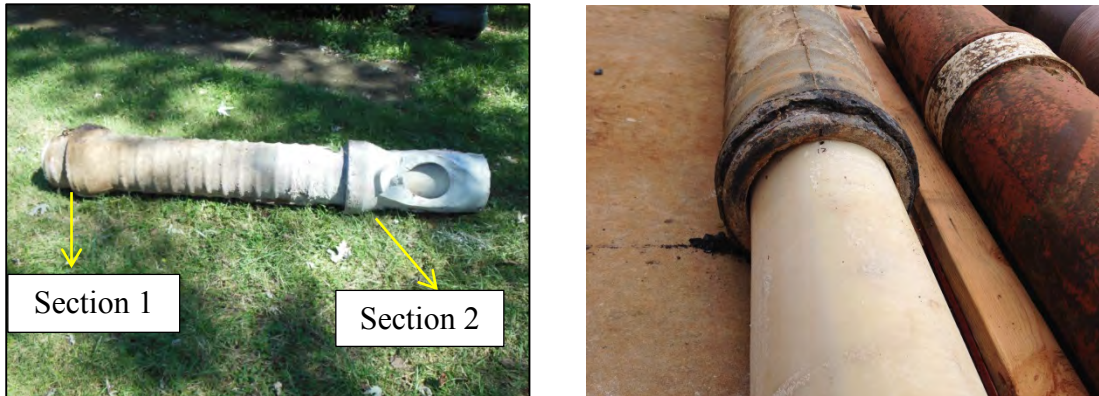
Figure C-34. Nashville Danby Dr.: Images of the HDPE Liner Section after Retrieval (left) and Taken in the TTC Laboratory (right)
