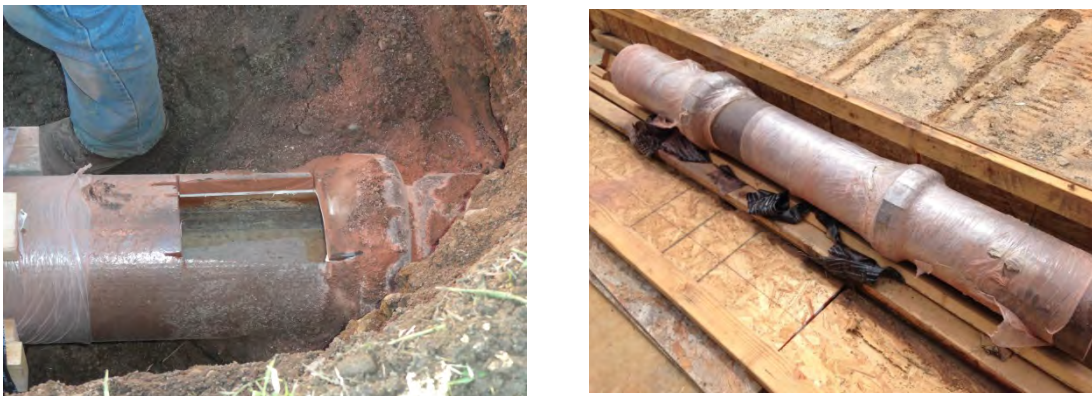
Figure C-1. Denver Ringsby Ct.: PVC Liner and Host Pipe during Retrieval (left) and at the Laboratory (right)
