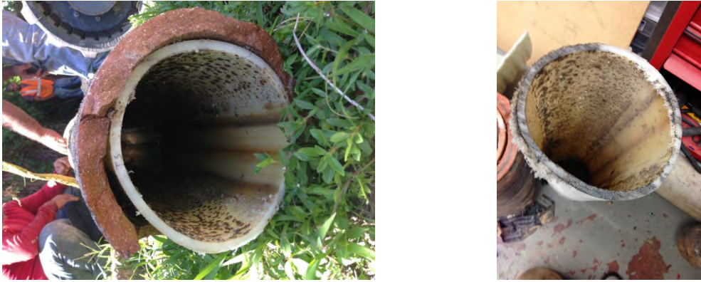
Figure C-25. Miami 114th St.: Images of the HDPE Liner Section in the Field (Left) and Prior to Testing (Right)
