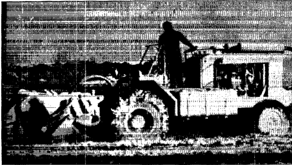
Figure 6-18. Mixing waste materials with stabilization/ solidification reagents in area mixing (Courtesy Soil Recovery).
