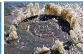
Aging Water Infrastructure
