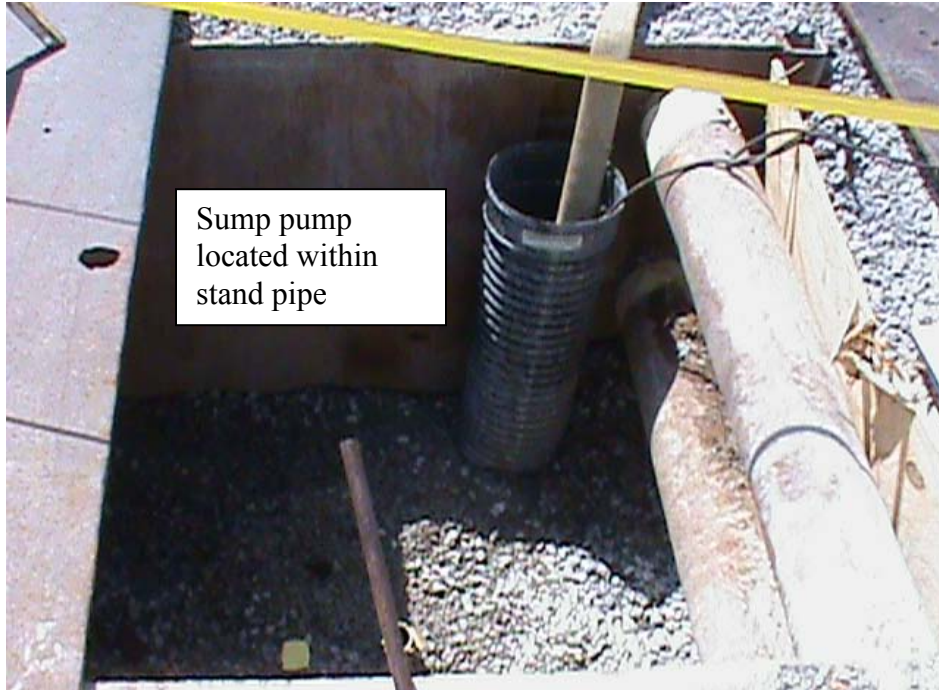
Figure 3-21. Sump Pump System for Simulated Leak Locations
