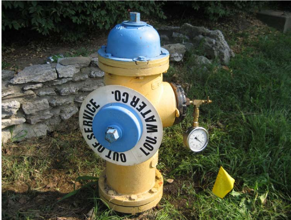
Figure 3-20. Monitoring Pipeline Pressure
