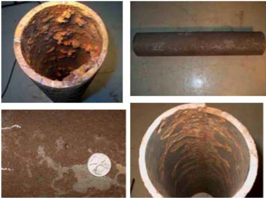
Figure 1: Photos of pipe with 4.2% measured loss
