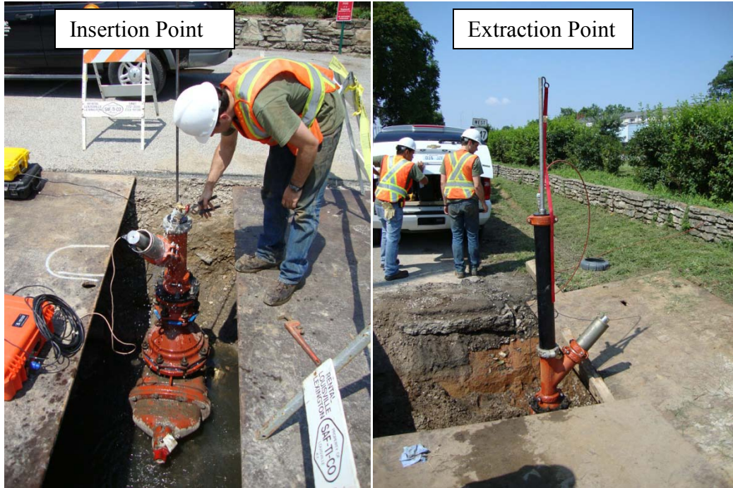
Figure 3-6. SmartBall™ Insertion and Extraction Tubes
