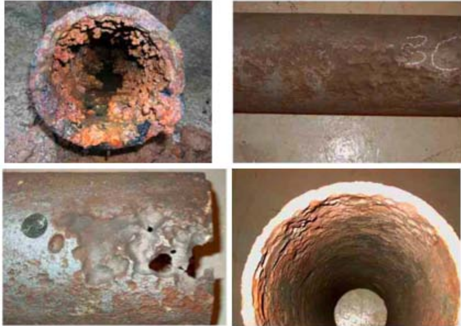
Figure 3: Photos of pipe with 47.3% measured loss
