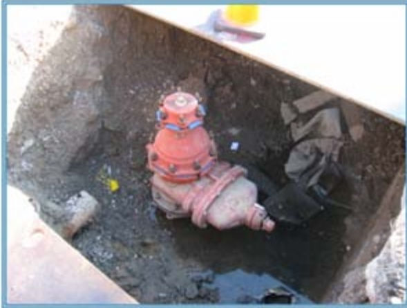
Sahara insertion site with valve and tap in Pit 1.
