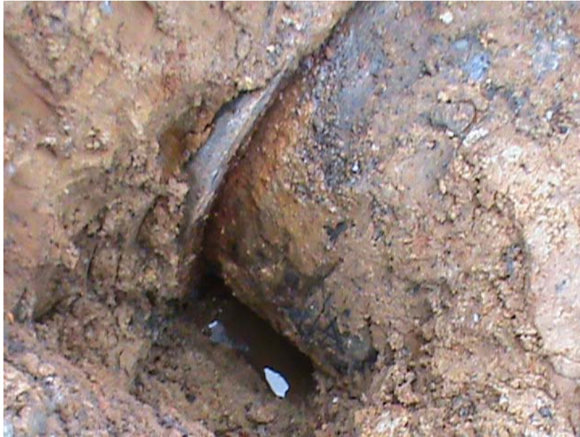
Figure 3-27. Leak ID L7 – Small Leak at Bell-and-Spigot Joint
