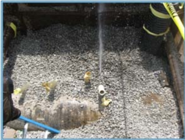
Valve creating a simulated leak in Pit 4.
