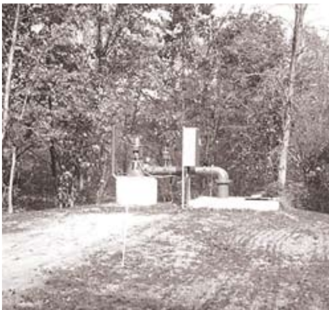
Public water supply well.
