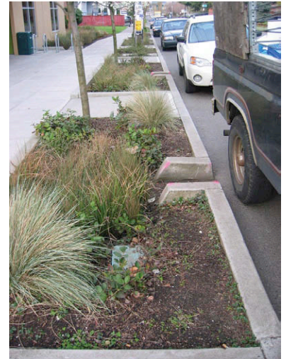
Curb cuts allow water from the street to flow into bioretention areas
