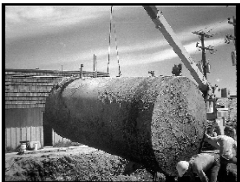
In 2004, there were 1,074 leaks from underground gasoline storage tanks in Indian Country.
