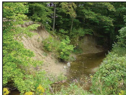
Note erosion of historic dredge spoils and poor instream habitat
