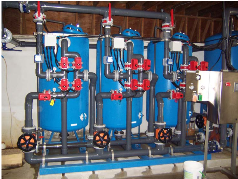
Figure 4-7. AD-26 Treatment System
