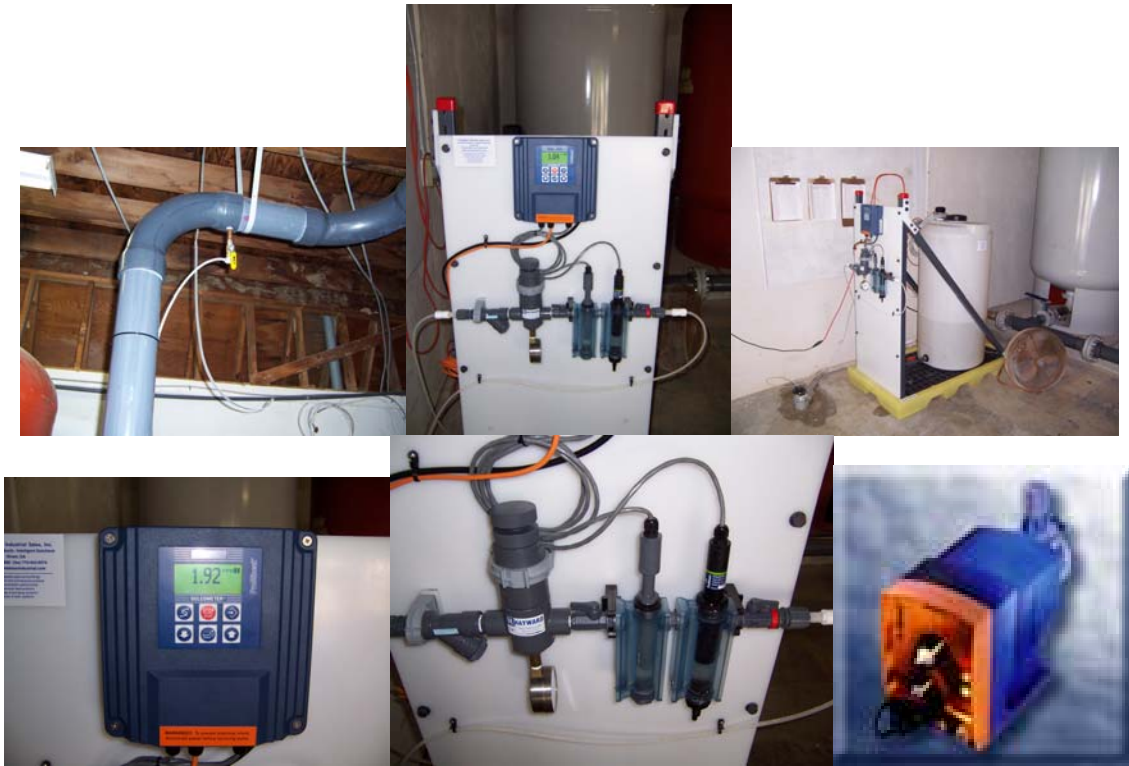
Figure 4-6. Chlorine Injection System
