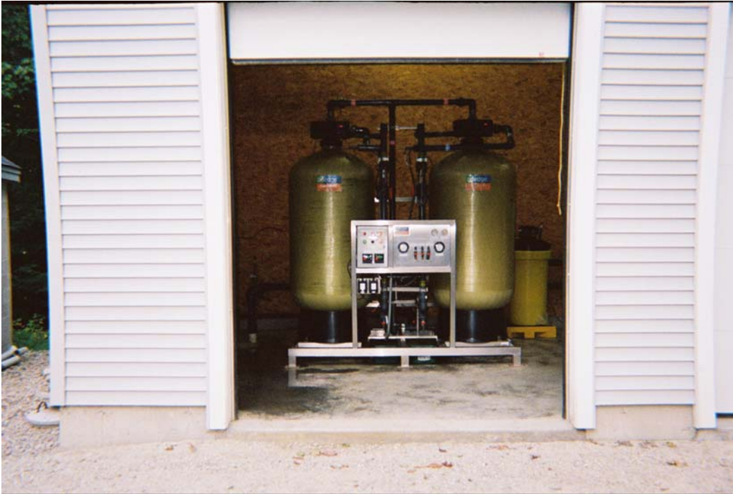
Figure 4-5. APU-100 Treatment System
