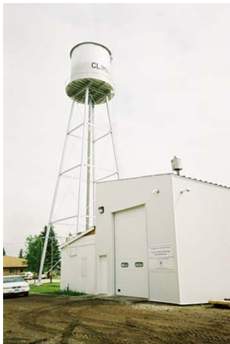
Figure 4-7. New Building Constructed Adjacent to the Pre-Existing Pump House and Water Tower
