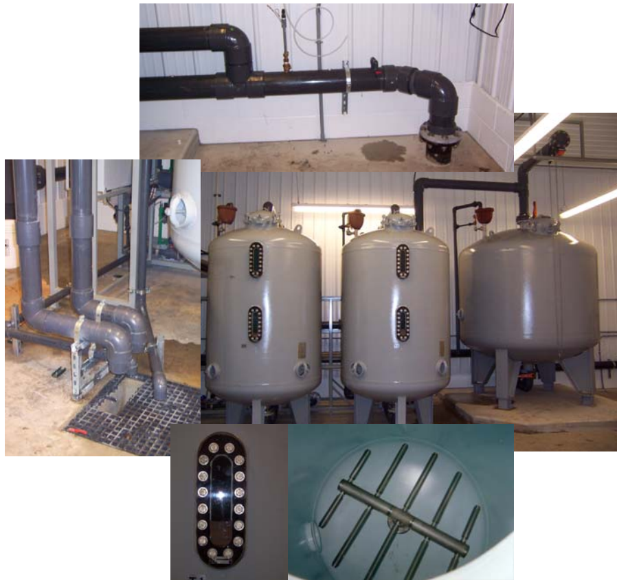
Figure 4-3. Treatment System Components (Clockwise from Top: Well No. 2 Entry and Bypass Piping; Two Filter Tanks and a Contact Tank; Filter Tank Laterals and Viewing Window; and Backwash Discharge Piping to Building Sump)
