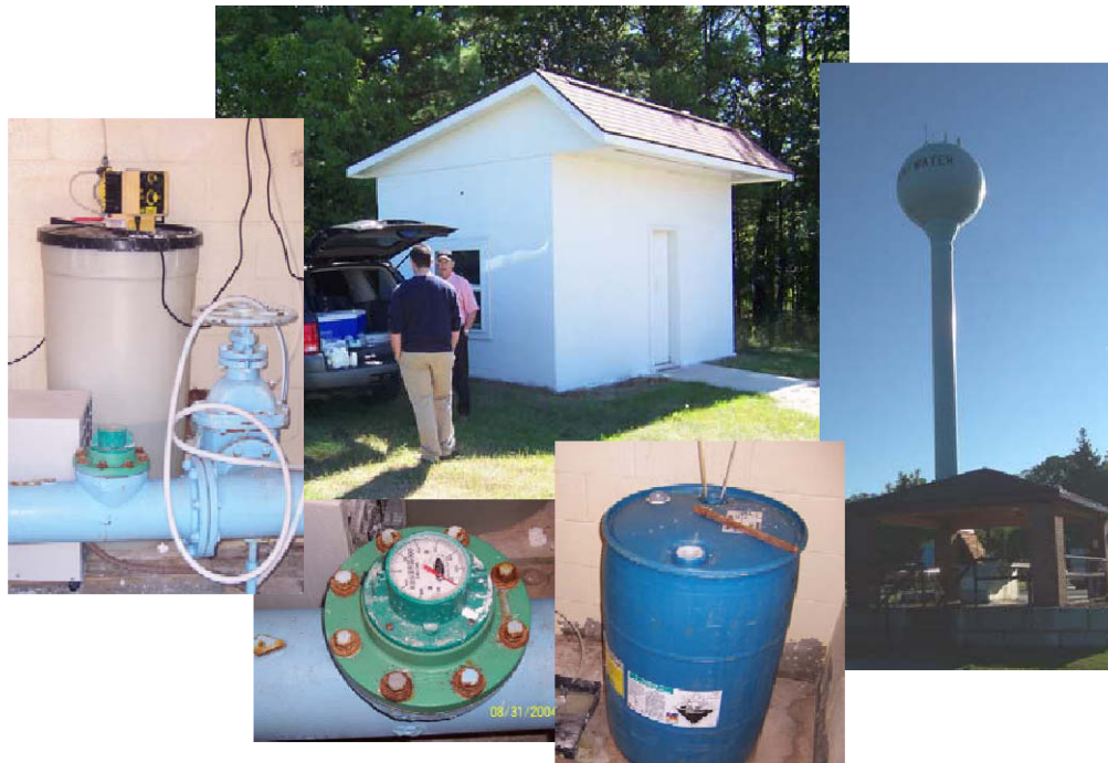
Figure 4-1. Existing Facility and System Components (Clockwise from Top: Well No. 2 Pump House, Water Tower, Polyphosphate Drum, Wellhead Totalizer, and Piping and Chlorine Addition Equipment)
