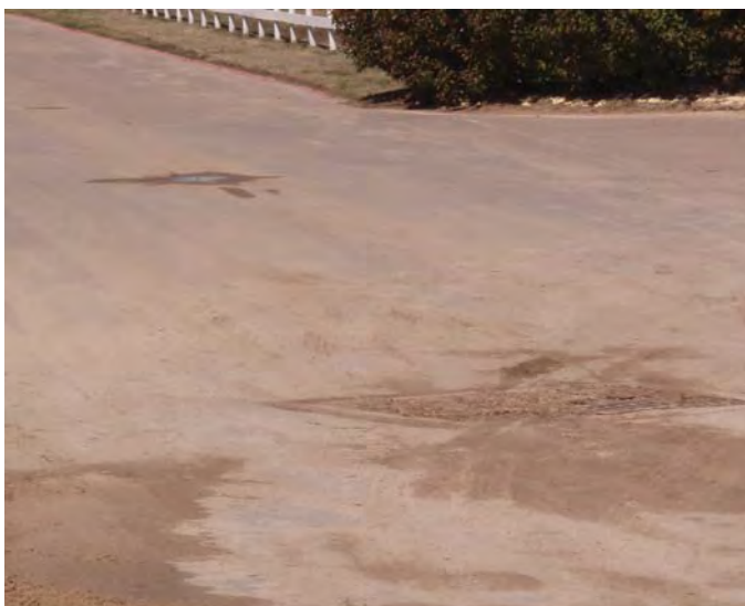
Photo 10. Storm water drain that collects runoff from the horse barn area and horse path areas.
