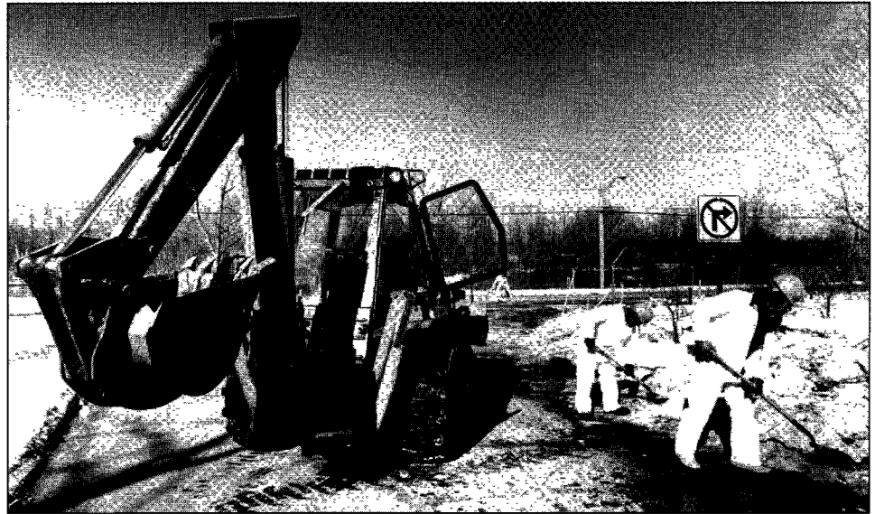
Man and Machine Cleanup often requires a wide array of techniques, from heavy machinery to workers' hands. The cleanup activities at Fulton Terminals included the removal of arsenic, barium, chromium and lead pollutants.
