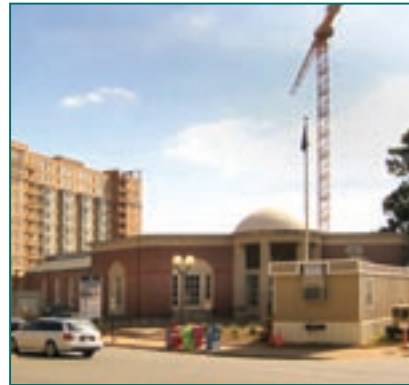
A construction crane rises above the Central Post Office redevelopment project in Arlington, Virginia.
