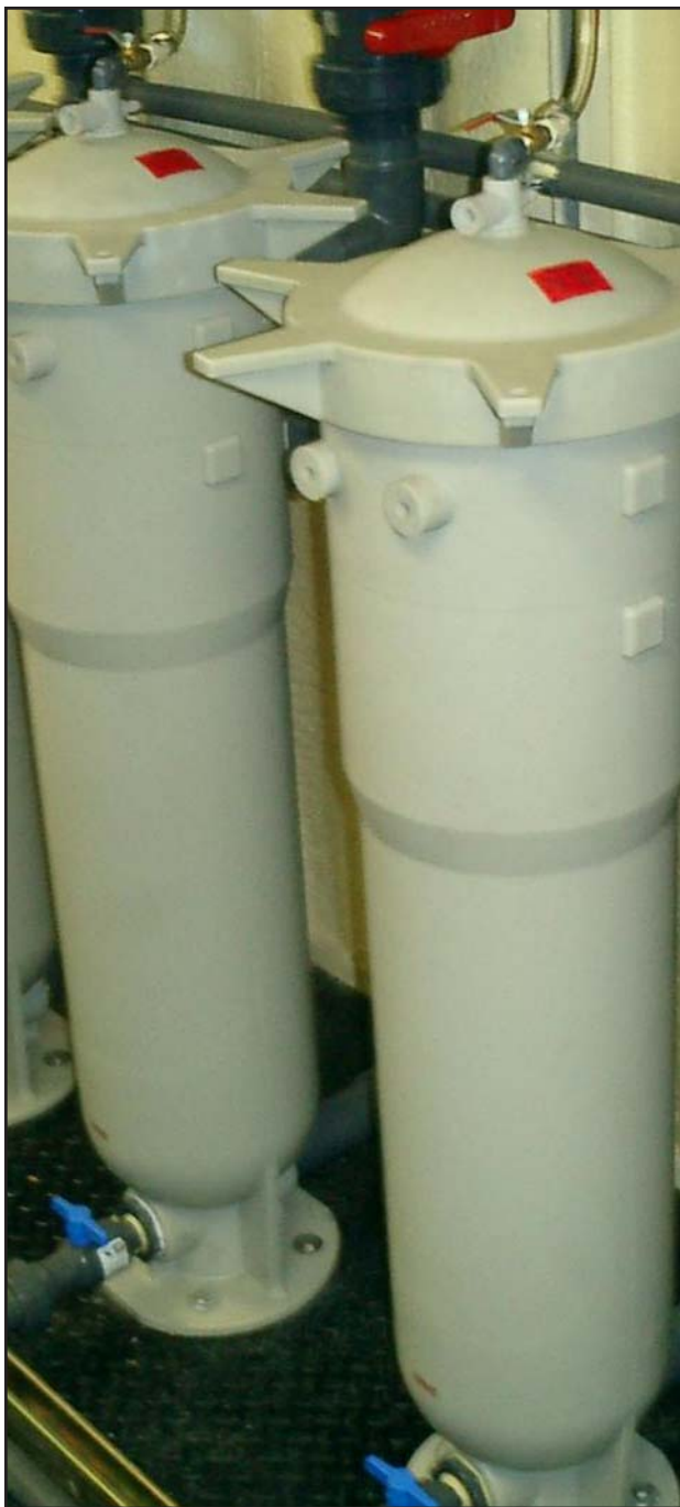
Bag filters for initial sediment removal.
