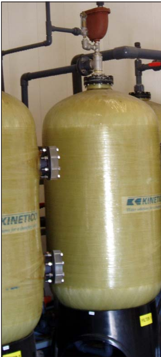
Pressure filter tanks for an arsenic removal system.
