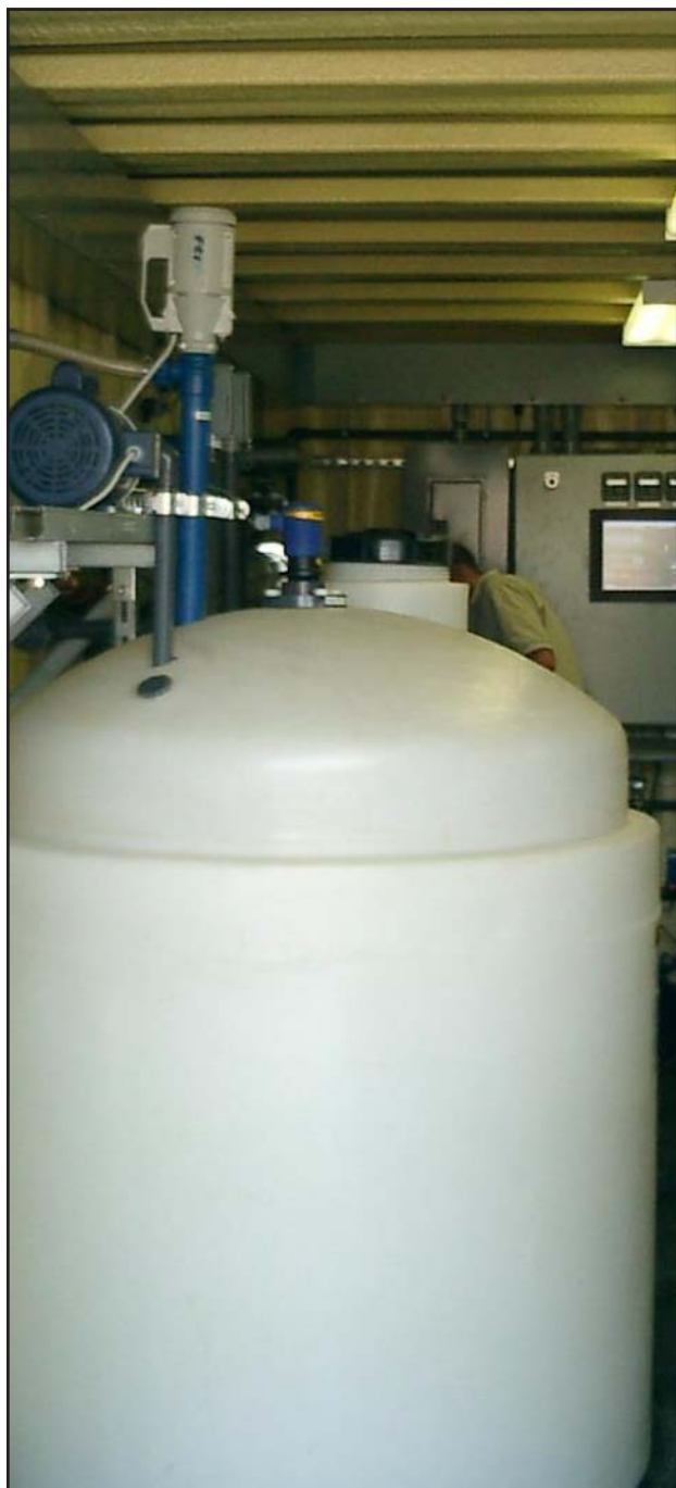
Chemical feed tank for an ion exchange system.
