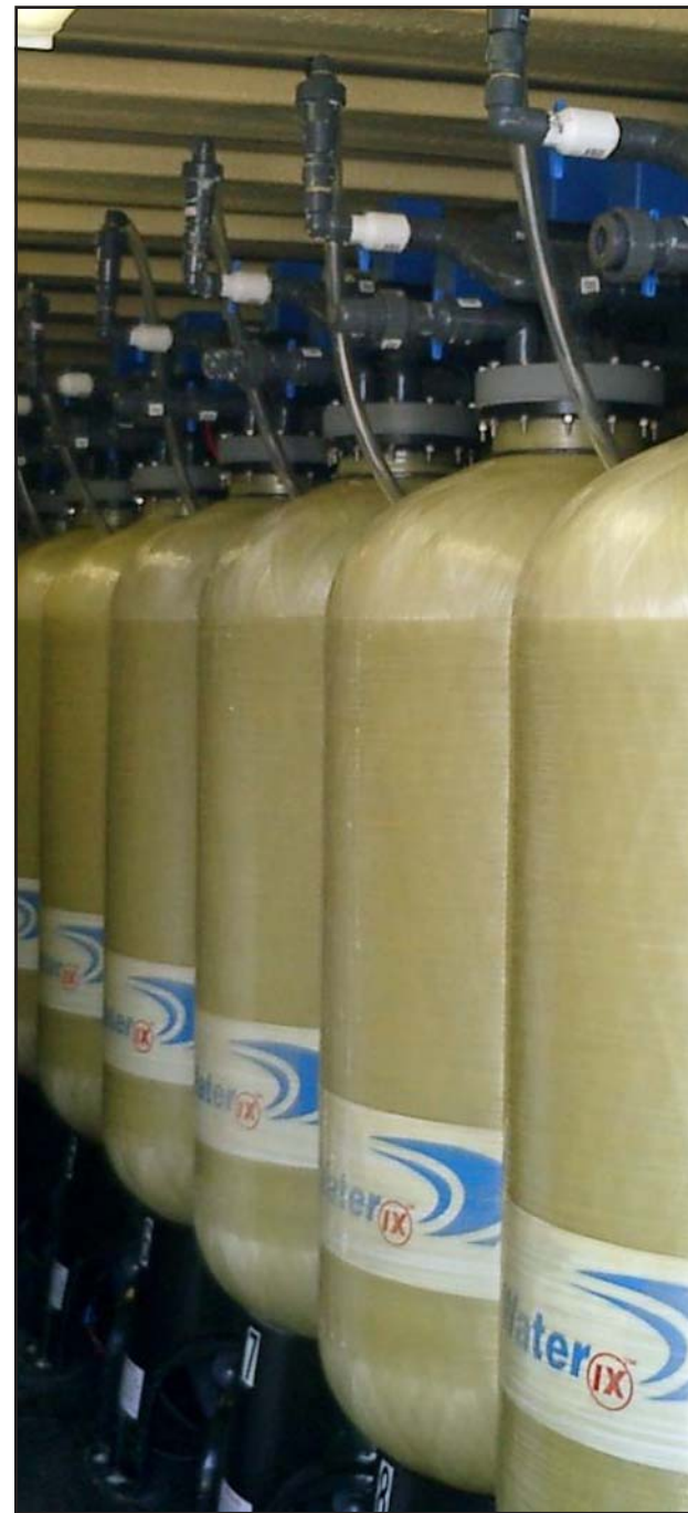
A row of ion exchange tanks in parallel.
