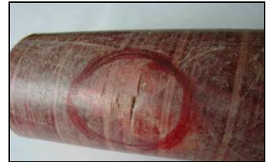
Fiberglass piping is cracked
