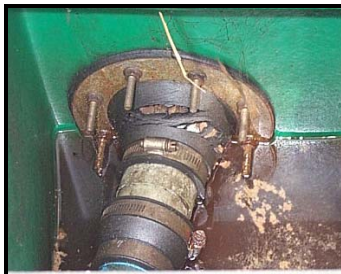
Sump penetration seals in poor condition
