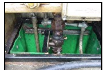
Contained dispenser sump
