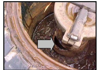
Spill bucket in poor condition – note the gap between the spill bucket and the fill pipe
