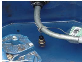
Liquid sump sensor
