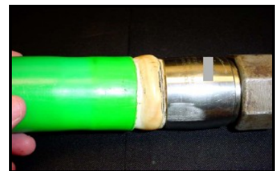
Flexible piping is bulging
