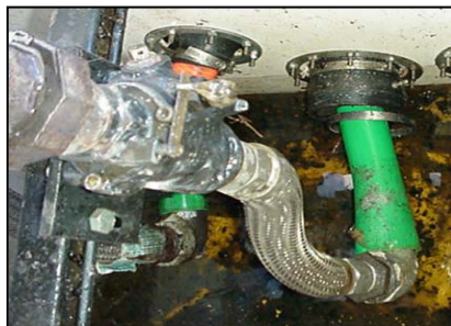
Metal flexible connector is twisted due to growth of flexible plastic piping
