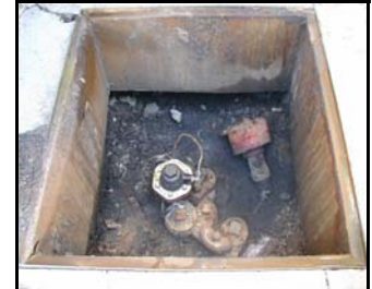
Uncontained turbine sump
