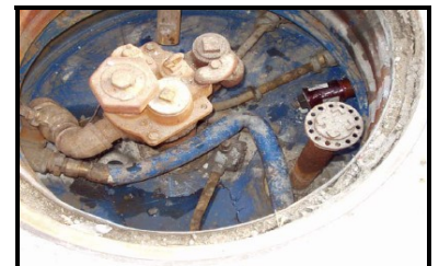
Flexible piping is kinked
