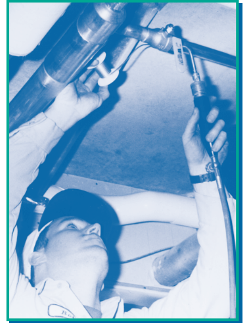
Pipefitter Bob Fitzgerald solders a connection in a new high-efficiency gas-fired water-based heating system at a 51-unit senior citizen home in Burlington, Vermont.
