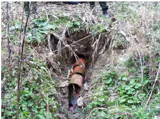
Land application on fields with sub-surface drainage tiles could result in a discharge.
