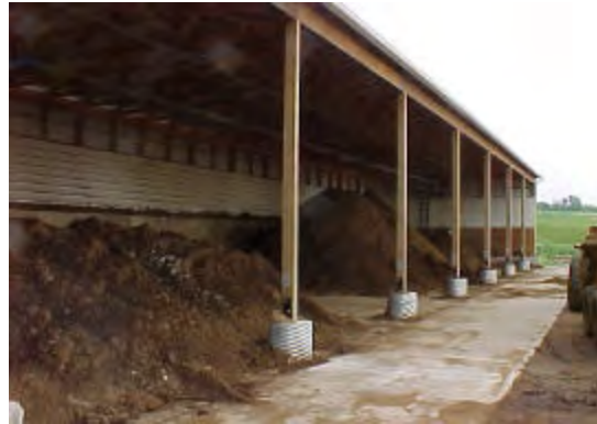
Covered compost and manure storage minimizes runoff.
