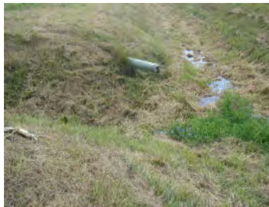
Uncontained discharges from manure storage ponds could contaminate surface water.
