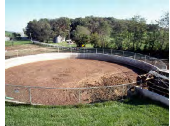
Tank storage with sufficient freeboard.
