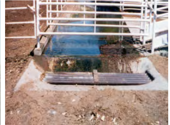
Concrete ditches (or well maintained grassed waterways) control effluents and carry it to a runoff holding pond.
