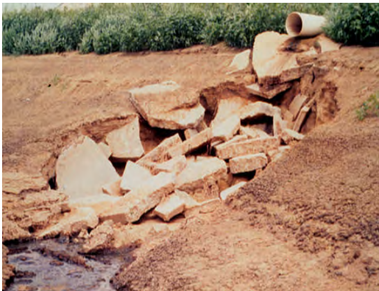
Earthen storage with eroded sidewalls could result in a discharge.
