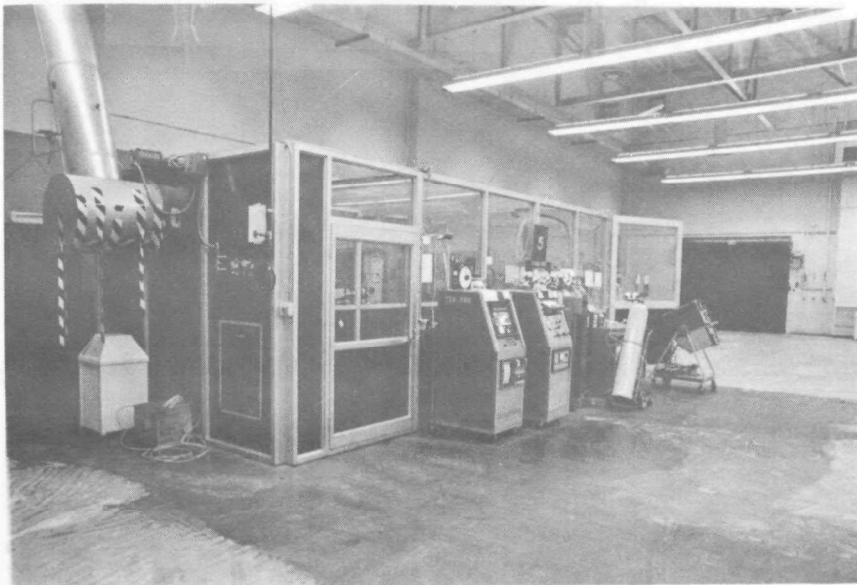
Figure 4-2 Evaporative Enclosure (rear view).
