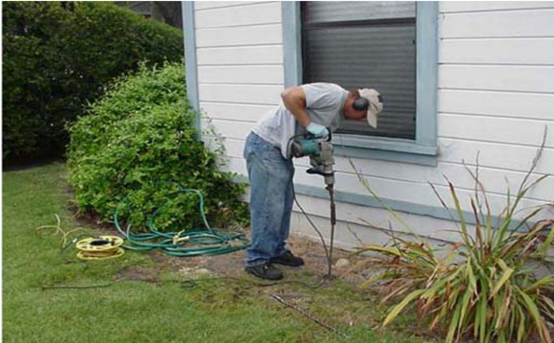
Figure 2. Installation of Soil Gas Probe Near a House. Soil gas probes are a primary method of collecting samples to measure soil-gas chemical concentrations.
