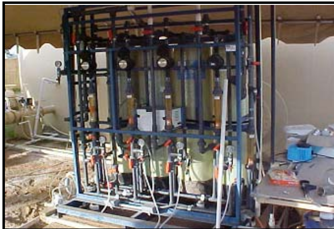
Figure 2: Scottsdale Pilot Testing Unit
