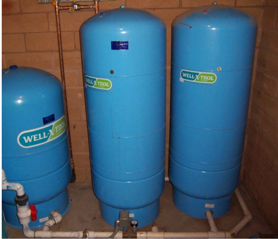
Figure 4-2. Pre-Existing Pressure Tanks
