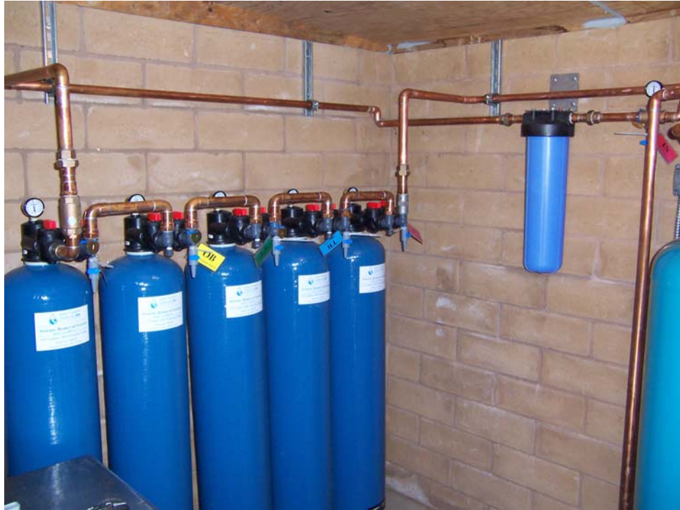
Figure 4-5. As/1200CS System with Oxidation and Adsorption Columns Shown Against Wall and a Sediment Filter Attached to Wall
