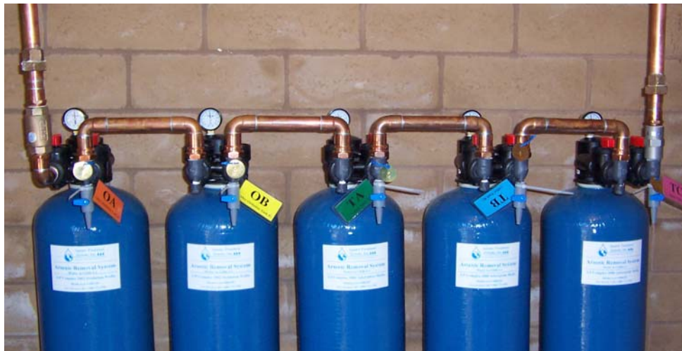
Figure 4-6. Close-up View of Oxidation and Adsorption Columns with Sample Taps and Labels
