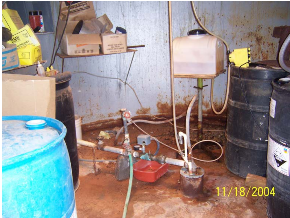
Figure 4-3. Pre-Existing Chlorine Addition System
