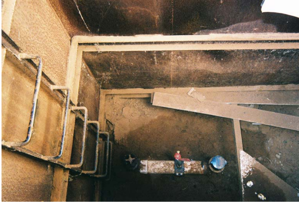
Figure 4-2. Vault Containing Supply Well Manifold, Sampling Tap, and Pre-Existing Master Totalizer
