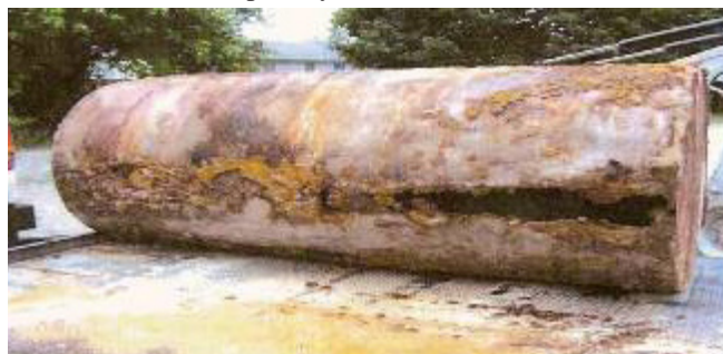
Excavated Leaking Underground Storage Tank
