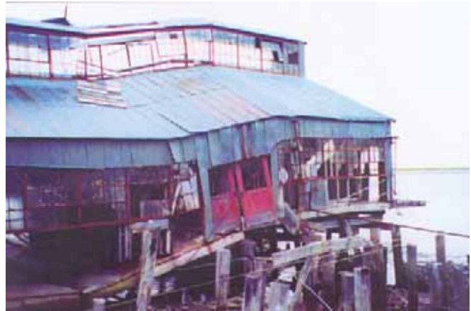
The main cannery building at Ugashik traditional village was collapsing before it was redeveloped as a flash-freezing facility.
