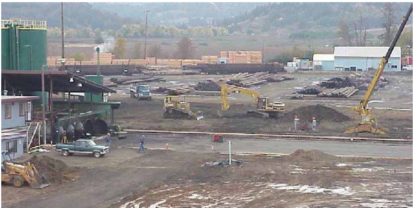
Wood preservatives with low environmental toxicity will be used at the Taylor Lumber and Treating site.
