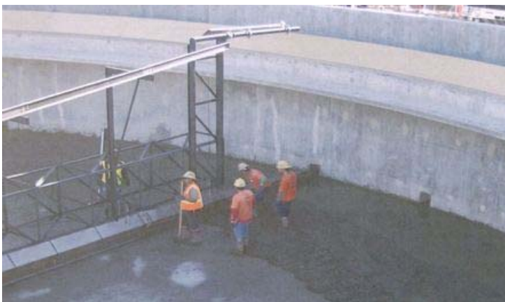
Photo 1: Construction of secondary clarifier, City of Petaluma, California (photo courtesy City of Petaluma).
