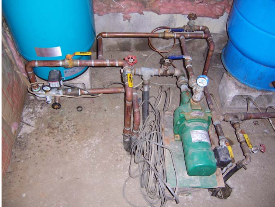
Figure 4-2. Pre-Existing Water Supply Pump, System Piping, and Hydropneumatic Tanks (shown in the background)
