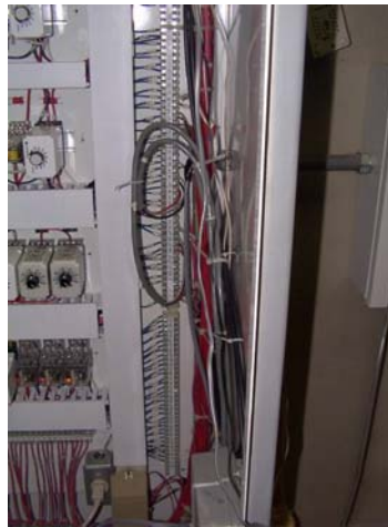
Figure 5-6. Picture of interface wiring.
