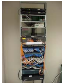
Figure 5-2. Picture of a fiber equipment rack.
