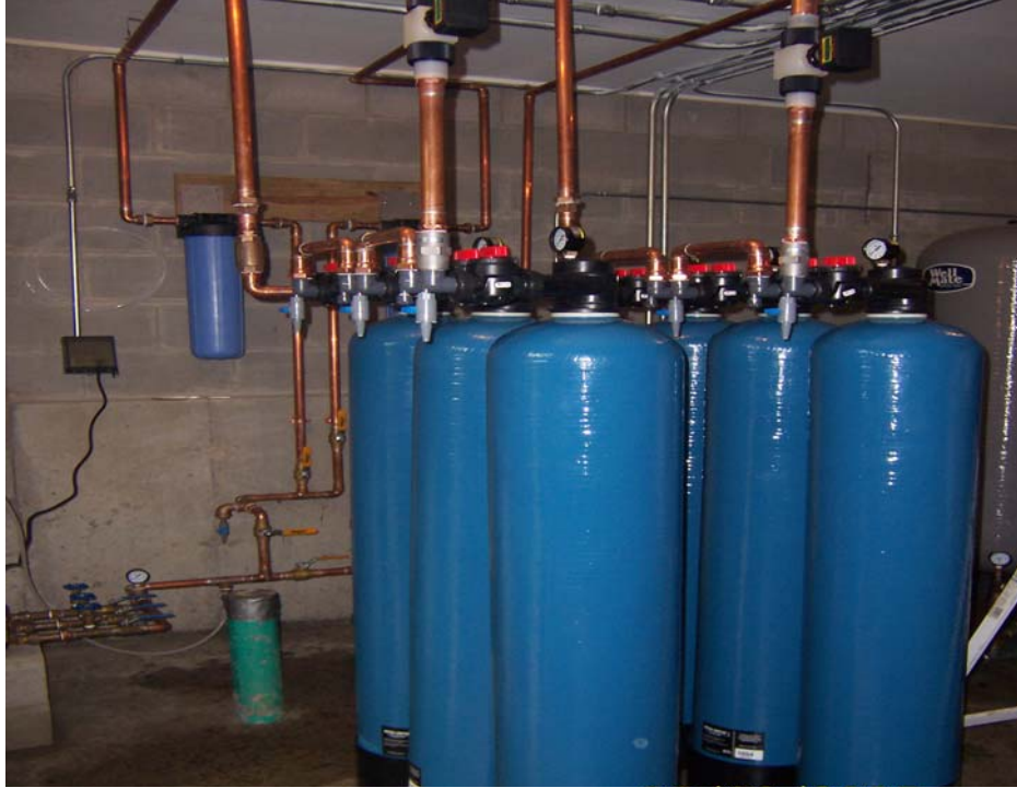
Figure 4-5. As/2200CS System with Adsorption Columns Shown in Foreground and Sediment Filters Attached to Wall
