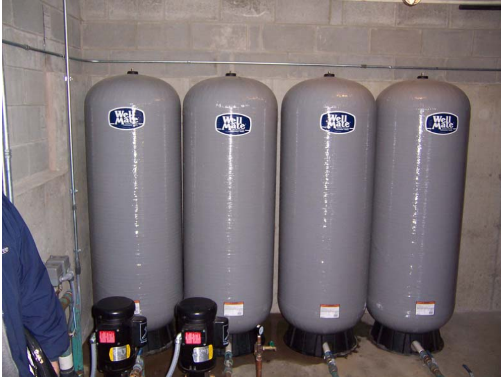
Figure 4-2. Pre-Existing Pressure Tanks and Booster Pumps
