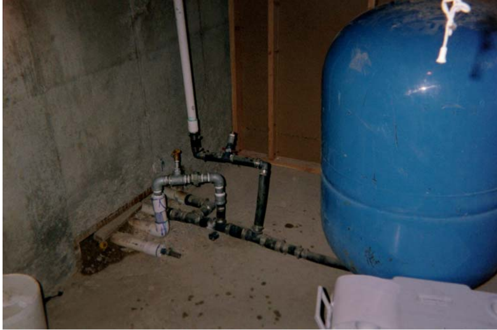
Figure 4-2. Plumbing from Well and Sample Tap at Sunset Ranch Development Site
