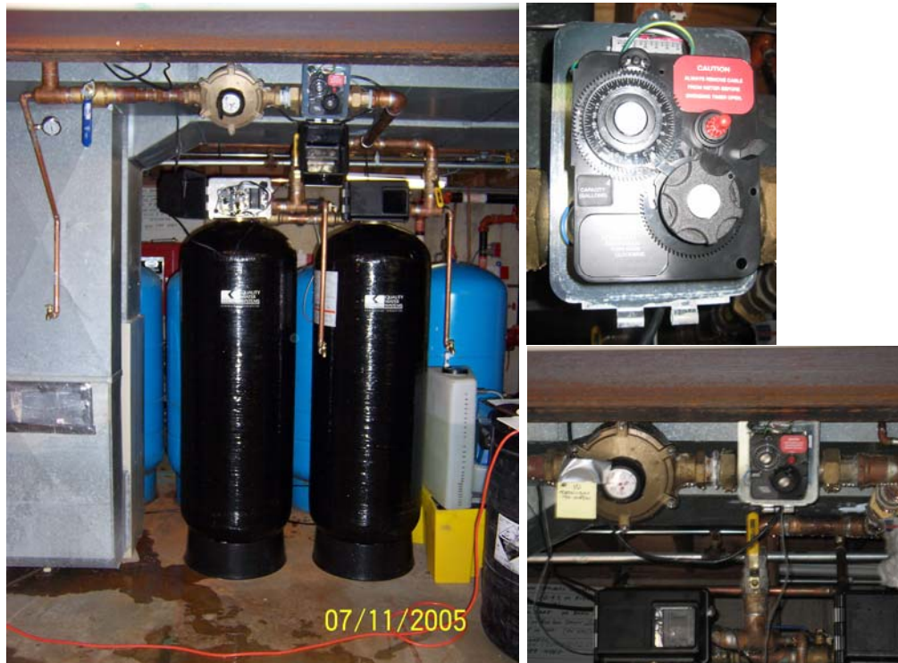
Figure 4-7. Macrolite® Pressure Filtration System (Clockwise from Left: Pressure Filters; Backwash Timer Assembly; Totalizer on Treated Waterline)
