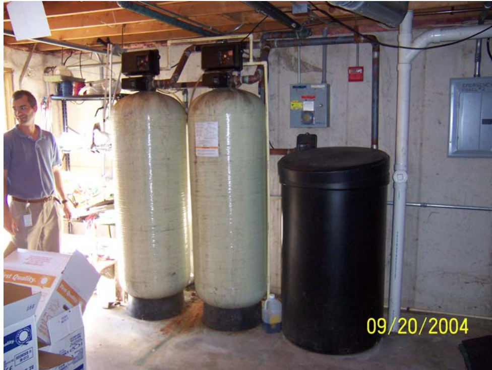
Figure 4-3. Preexisting Softener System
