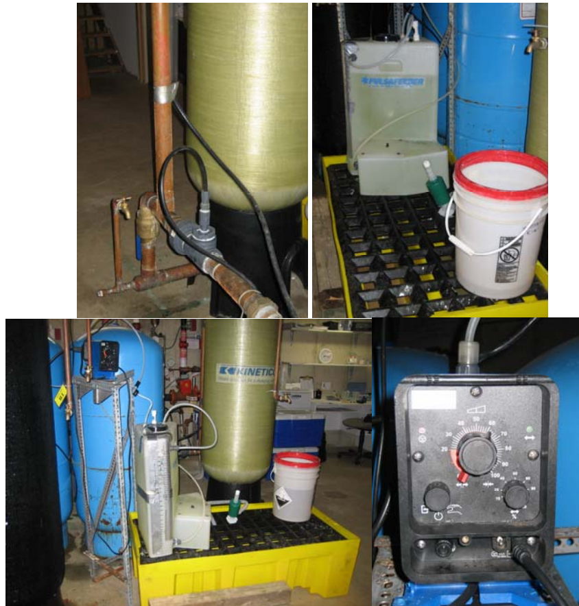
Figure 4-5. Chlorine Addition System
