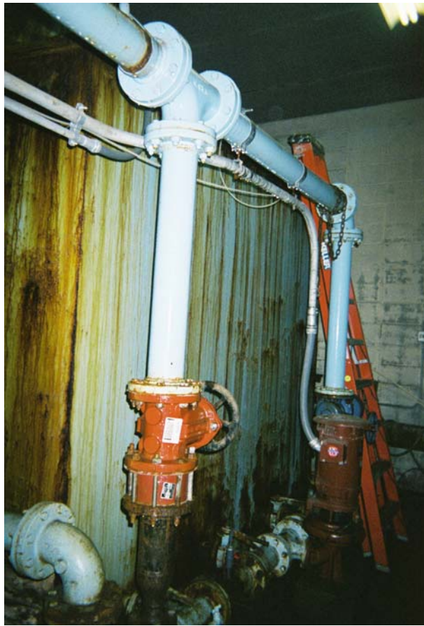
Figure 4-2. Preexisting Filtration System at Sabin, MN
