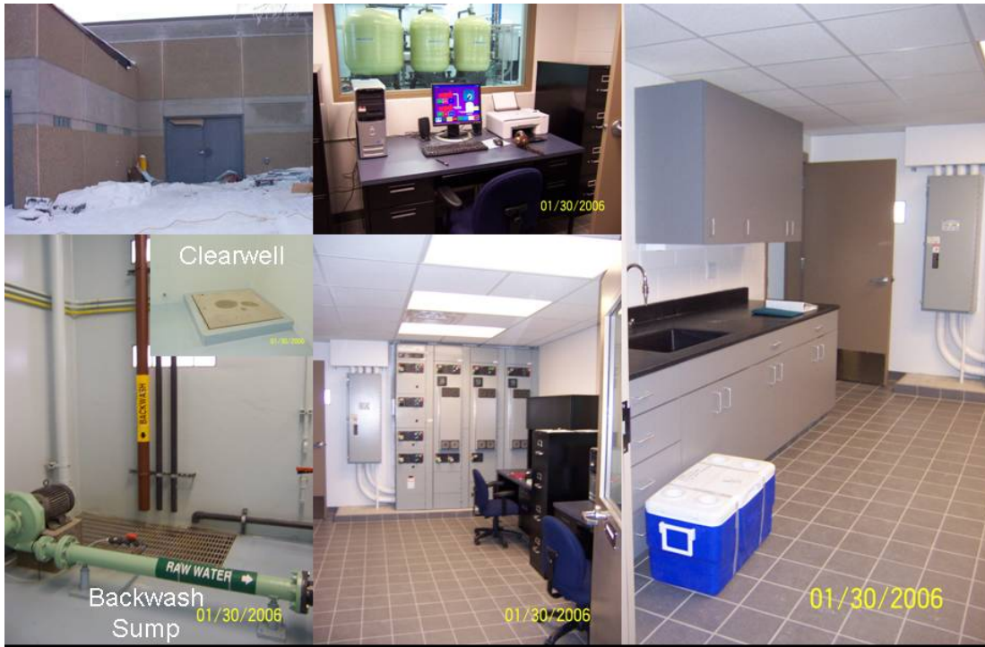
Figure 4-6. New Building and Associated Infrastructure (Clockwise from Top, Left: New Building, Adjacent Office/Laboratory Area, and Electrical Control Panel, Clearwell Lid [Inset], and Backwash Sump)
