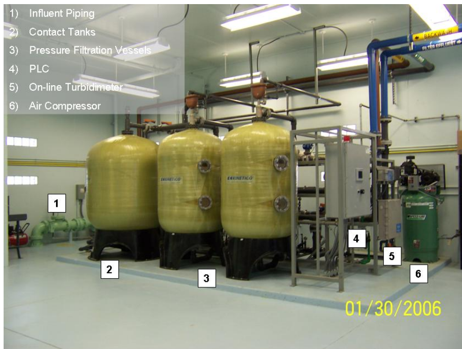
Figure 4-5. Treatment System Components
