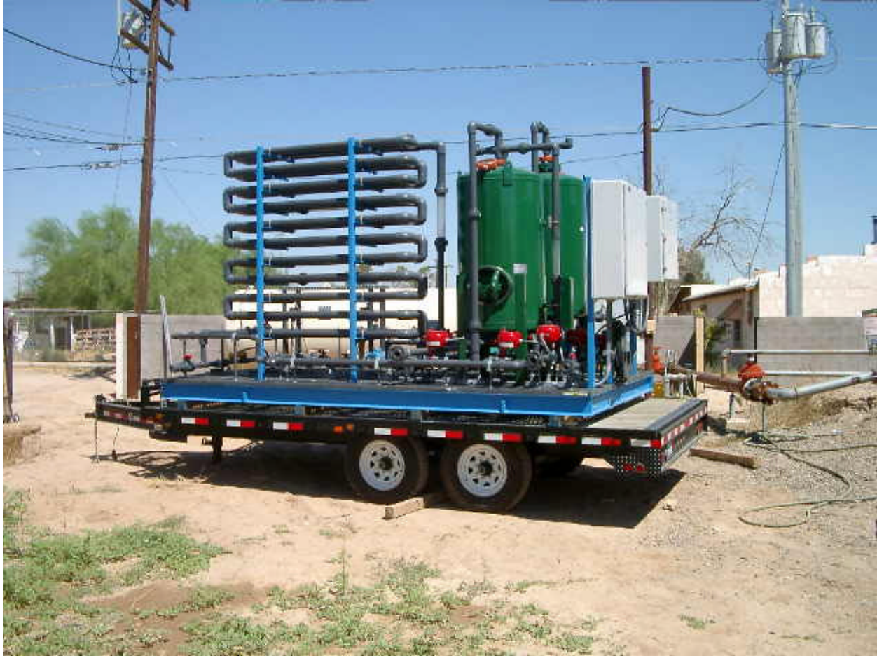
Figure 2-2. KemLoop System skid mounted unit photograph.
