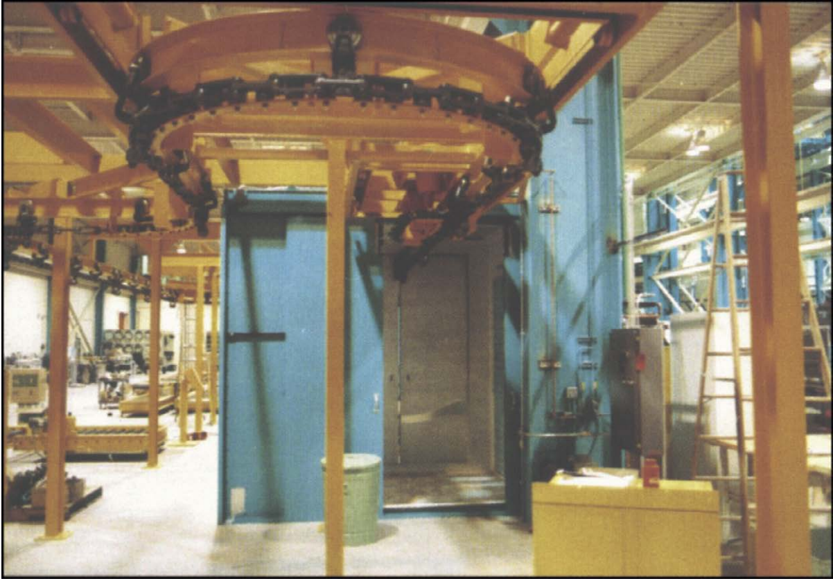
Figure 2-3. A Conveyorized Paint Finishing Booth
