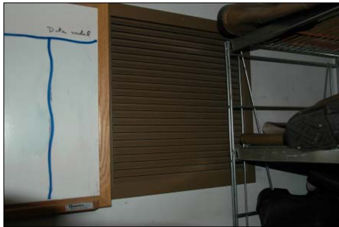
Figure 8 Equipment Room Vent (inside equipment room 41 \mu\text{g}/\text{m}^2 PCBs)
