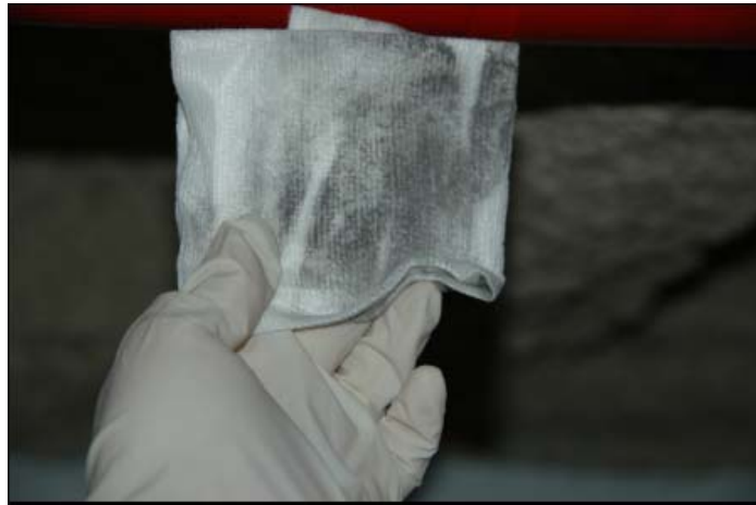
Figure 10 Sprinkler Pipe Parking Level 1 (60 \mu\text{g}/\text{m}^2 PCBs*)
