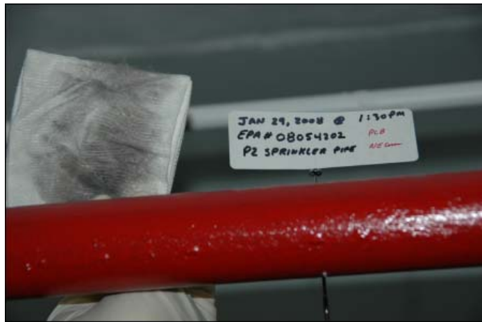
Figure 11 Sprinkler Pipe Parking Level 2 (26 \mu\text{g}/\text{m}^2 PCBs)
