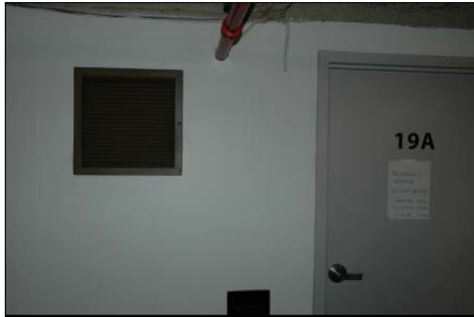
Figure 7 Equipment Room Vent (outside equipment room 133 \mu\text{g}/\text{m}^2 PCBs)
