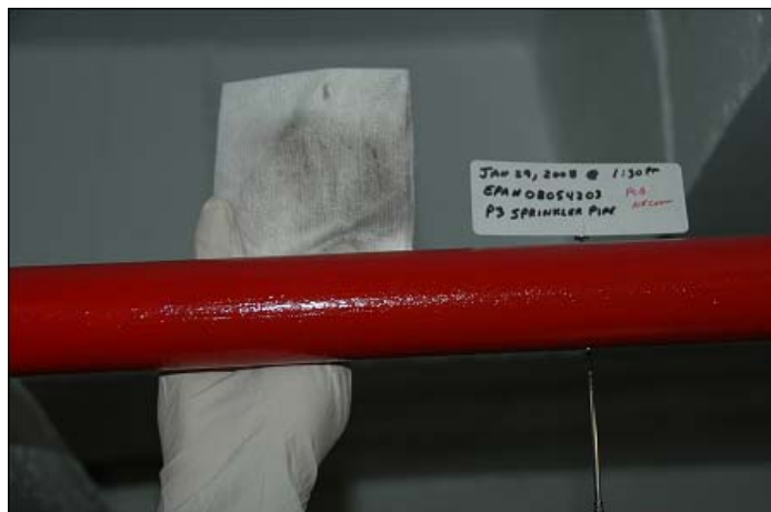
Figure 12 Sprinkler Pipe Parking Level 3 (14 \mu\text{g}/\text{m}^2 PCBs)
