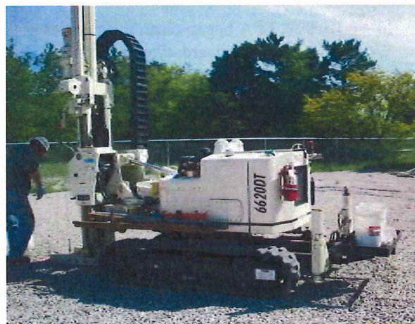
Equipment such as this Geoprobe may be used to collect samples in the Little Scioto River.
